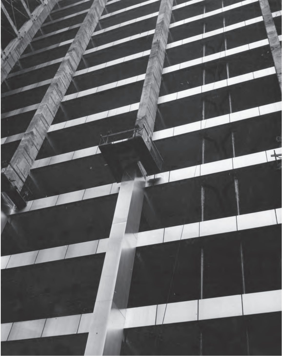
Figure B.5: View Looking Upward - East Wall of Main Building, Showing Stainless Steel Column Covers and Spandrel Panels. Source: Kaufmann and Fabry Co., SOM Archives, 3/20/1957.
