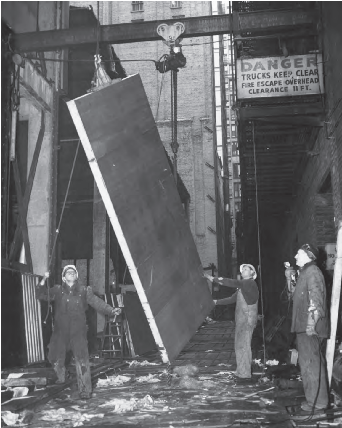
Figure B.6: Stainless Steel Covered Panel (5'-1"x13'-0"x5"; 3500 lb.) Being Turned on End, Without Touching Ground, Preparing to Hoist to Upper Floor Level of Service Tower. Source: Kaufmann and Fabry Co., SOM Archives, 5/16/1957.
