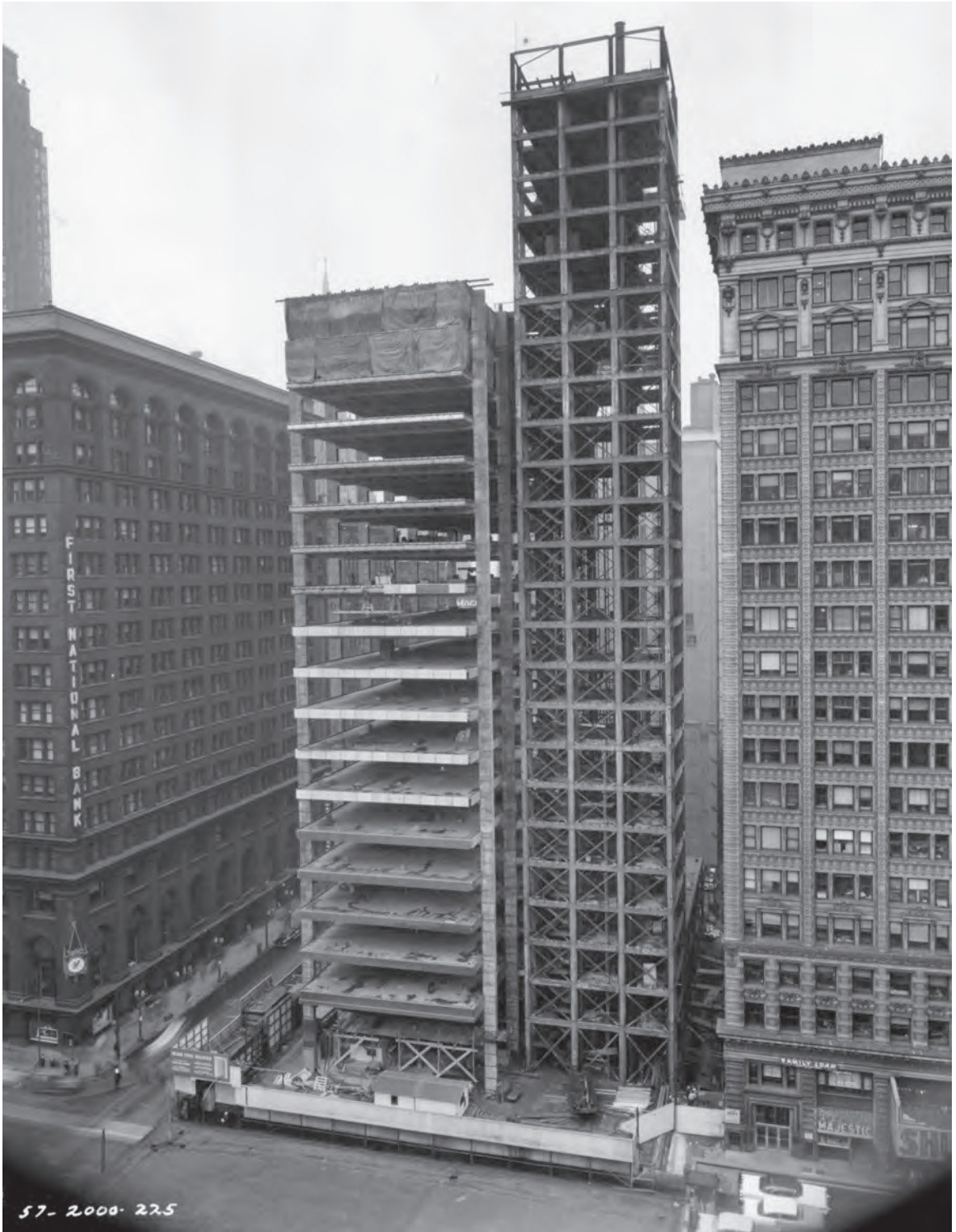
Figure B.7: Architectural View No. 43 Looking N at Building. Source: Kaufmann and Fabry Co., SOM Archives, 2/21/1957.
