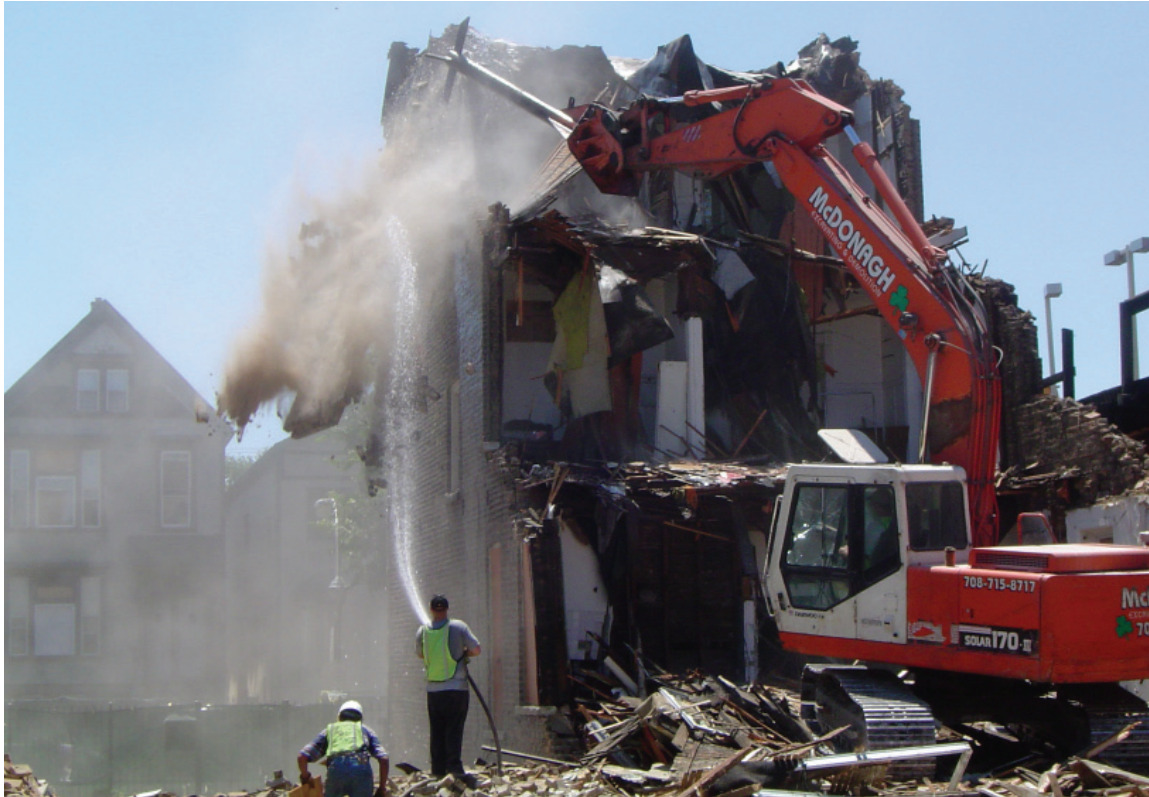
Image 5.1: A hydraulic excavator vanquishes a brick three-flat in the Lake View community area at 936 West Fletcher Street; 2005
