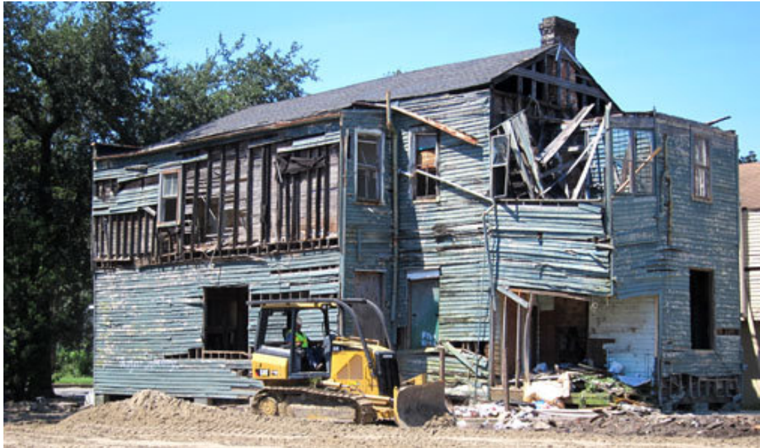
Figure A5. Structurally Unsound Blight. Source: http://photos.nola.com/
