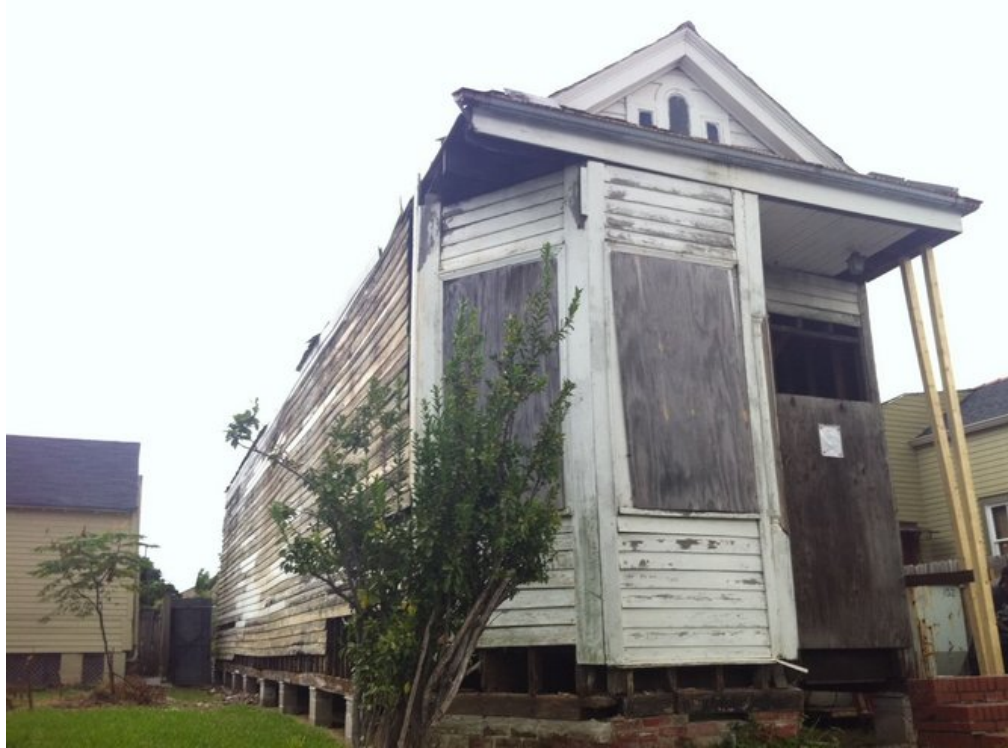
Figure A3. Boarded Blight. Source: http://photos.nola.com/
