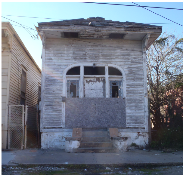
Figure 22. 1618 Annette. This property sold at auction in June 2010. Nearly two years later, it remains blighted. Photograph taken by author, January 2012.
