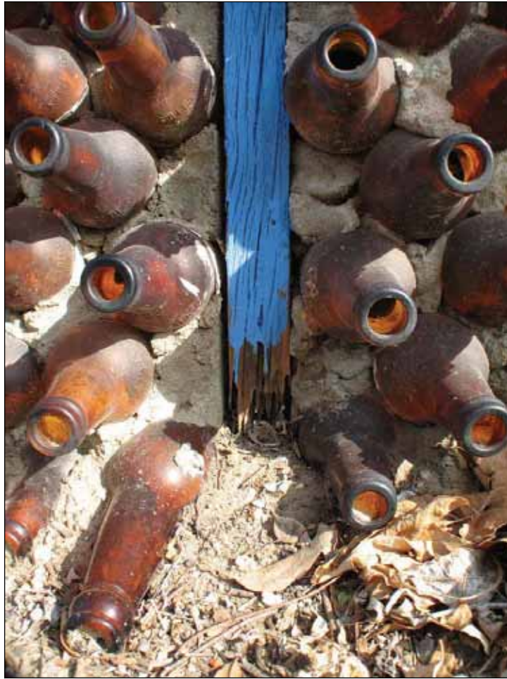
Figure 7.14: Round House wood framing, rot and termite damage due to direct contact with damp ground. (TSD 2007)
