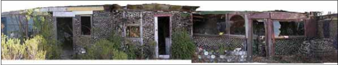
Figure 6.2: Ortho-rectified montage of School House, Shell House and Third Pencil House. (R. Eppich 2007)
