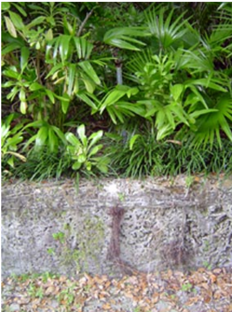
Fig. 35 – Water spigot and damaged stone cladding on a retaining wall planting. Notice the root systems of the plants penetrating through the stone. (summer 2003)
