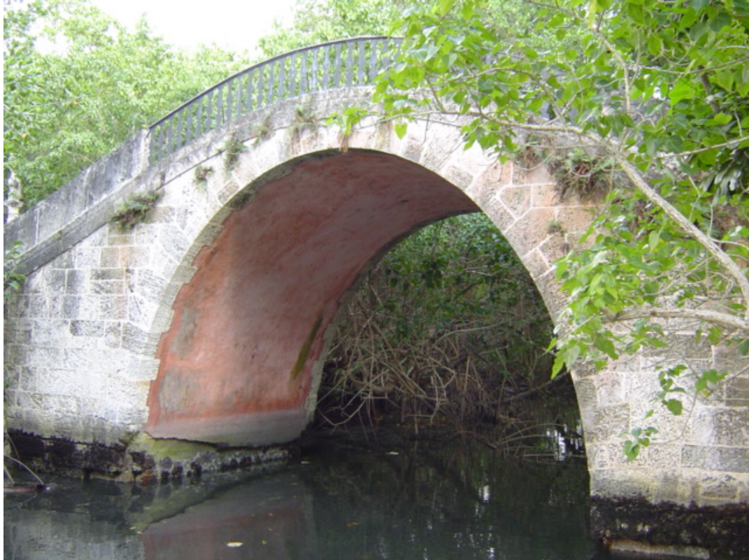
Fig. 14- Peacock Bridge connecting link between the two sides of the Marine garden over the canal. (Summer 2003)
