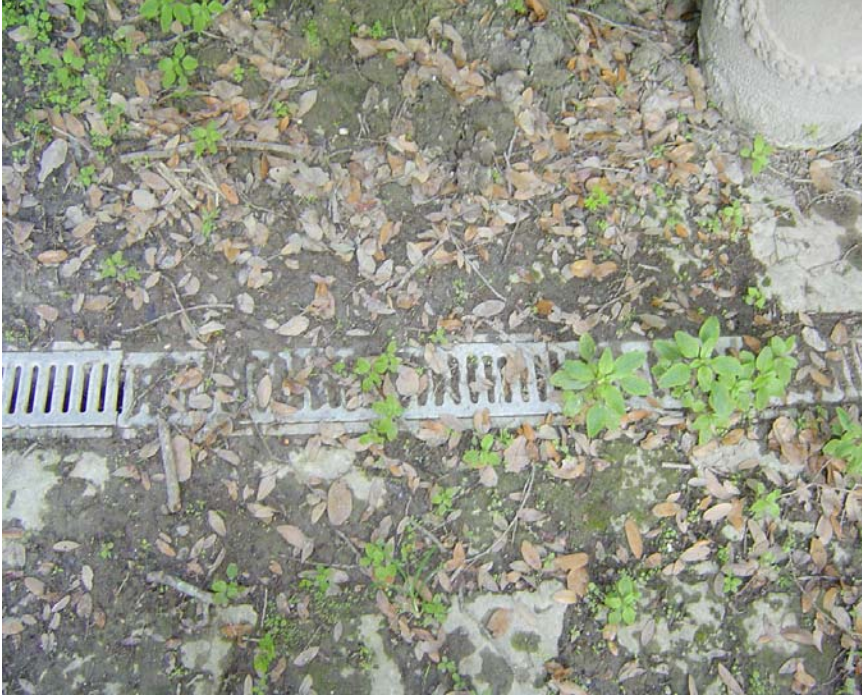
Fig.33 Clogged drains in the Marine garden, (summer 2003)
