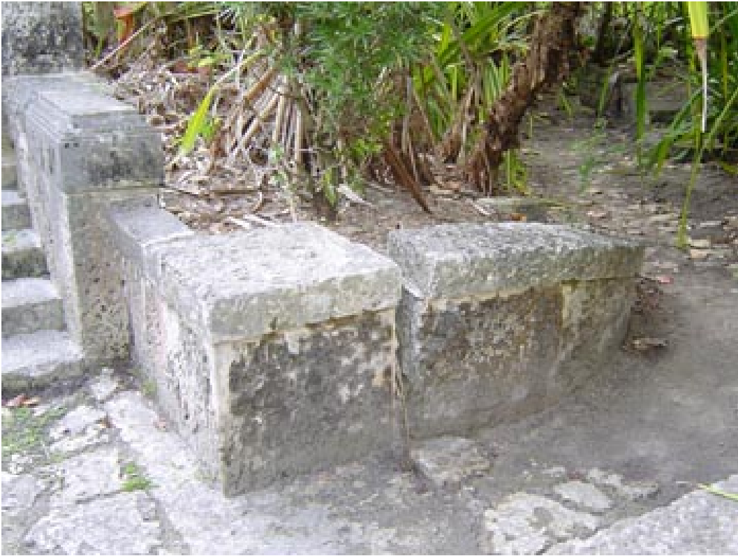
Fig. 34 – Dislodged retaining wall block due to overgrown root systems (summer 2003)
