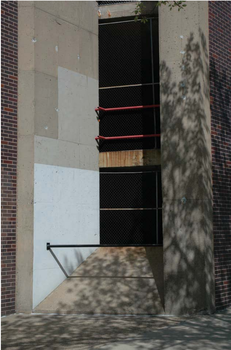
Image 38: Painted sections of exposed concrete at Walnut Street garage
