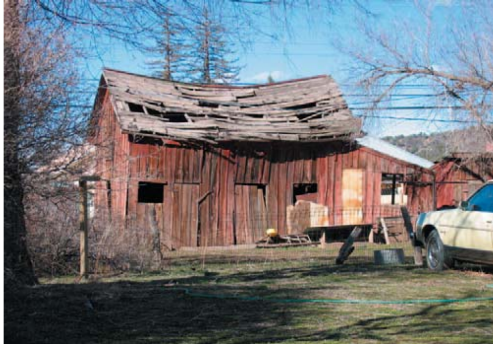
Figure 43-Small Wooden Structure in Disrepair, Mancos, 2005
