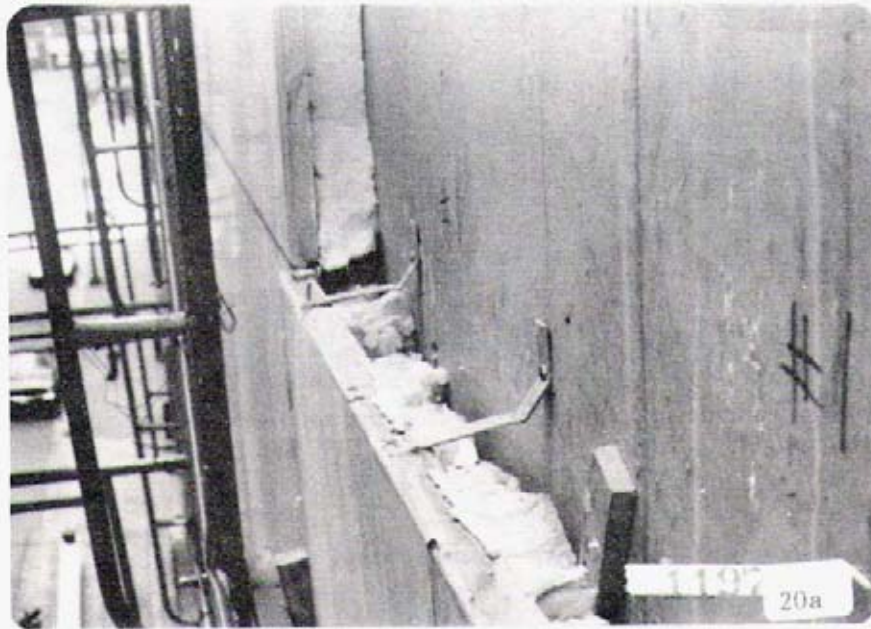
Figure 1.6 Bending anchor caused by lateral loading. (Photo from Bortz, et al., 27.)
