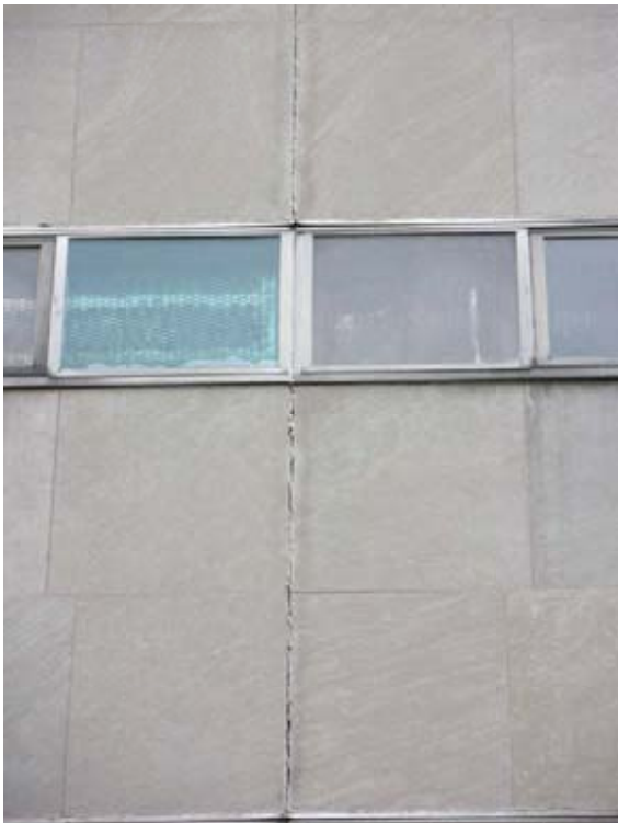
fig. 11 Expansion joint on Parkway façade from 1978 renovations, photo by Anny Su, November 2005
