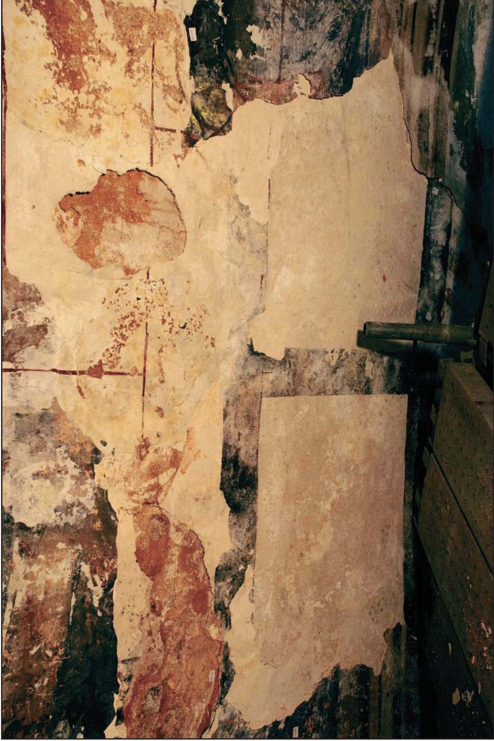
Figure 30: Detail (A6-2) Ashlar motif evident in the dome, Campaign A (Source: C. Silva, 2006)
