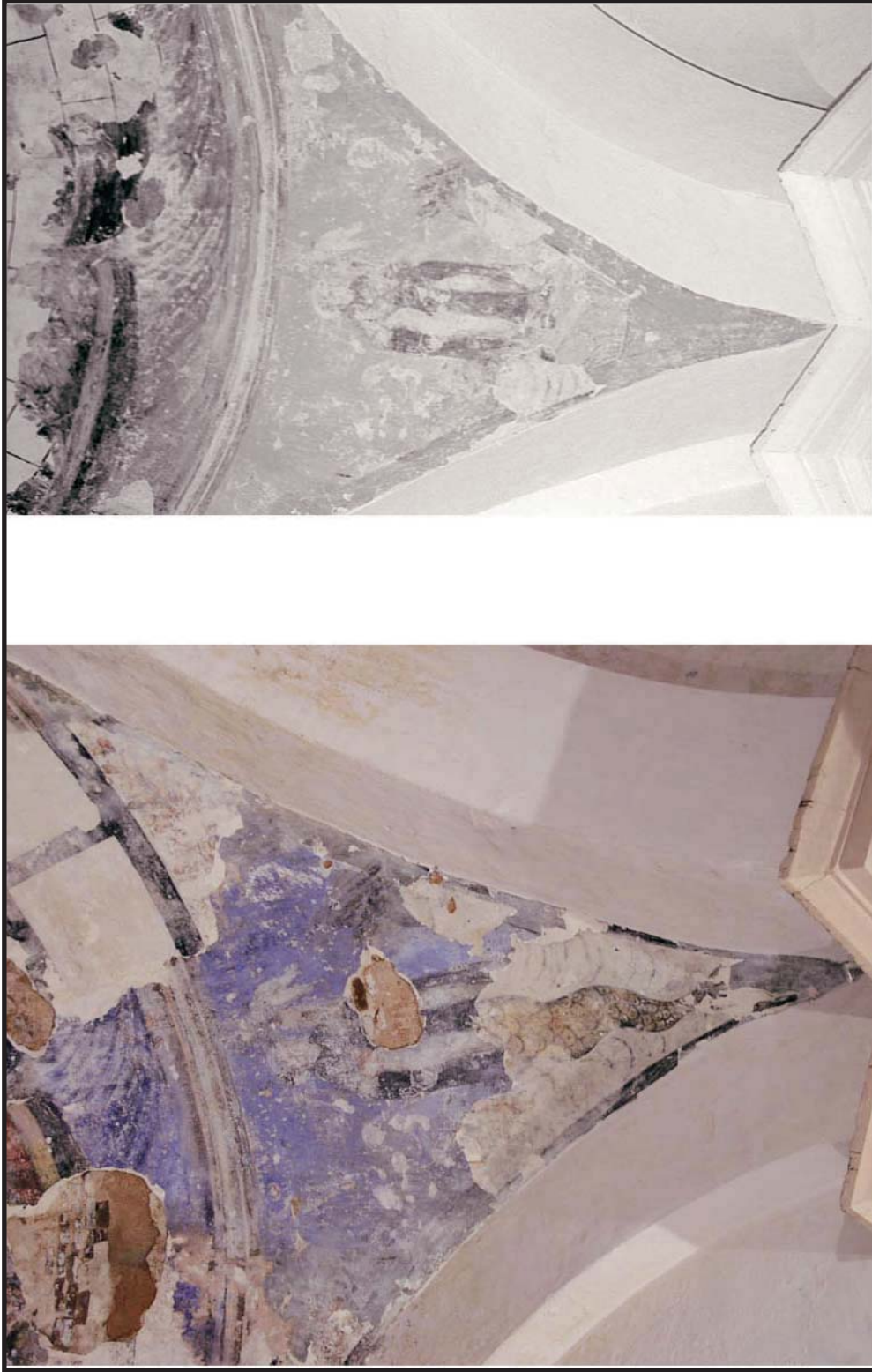
Figure 17: Photographic comparison of Pendentive 1, on the left is a 2004 image and on the right, an image taken in 1981. Note the deterioration in terms of areas of loss and image legibility over a twenty year time span. (Source: Pantel y del Cueto & Associates)
