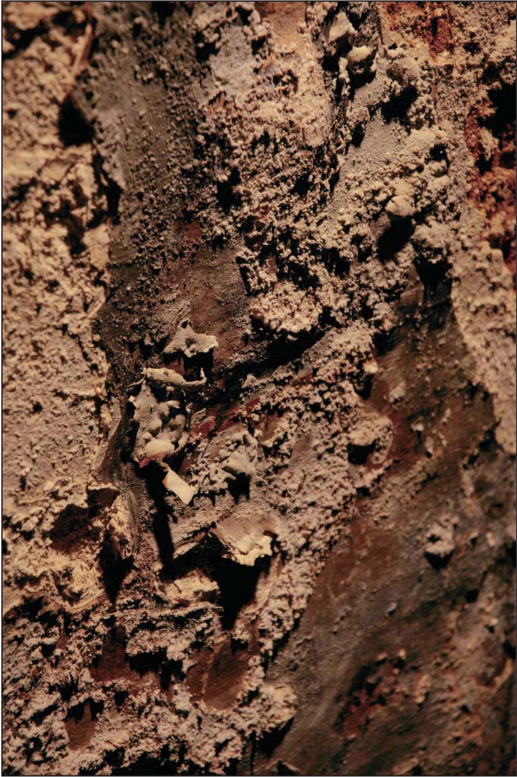
Figure 66: Detail (A8-8) Image of surface conditions: blistering, flaking, and salts (Source: C. Silva, 2006)
