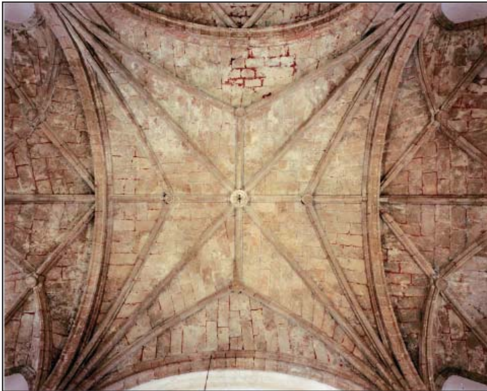
Figure 3: Stelliform groin vaulted ceiling of the Sanctuary. (Source: Pantel y del Cueto & Associates, 2002)
