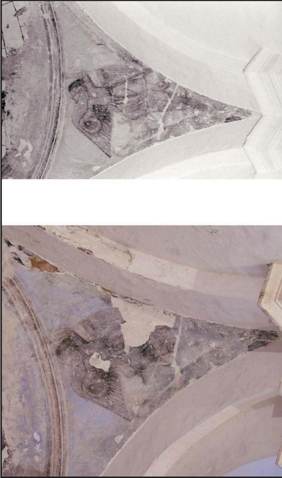
Figure 23: Photographic comparison of Pendentive 4, on the left is a 2004 image and on the right, an image taken in 1981. Note the deterioration in terms of areas of loss and image legibility over a twenty year time span. (Source: Pantel y del Cueto & Associates)
