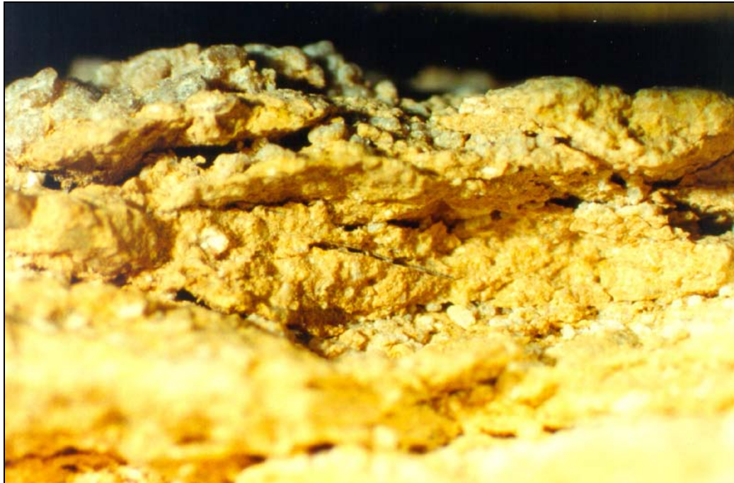
Figure IV.16 Flaking and delamination of the stone surface caused by salt crystallization. Sample 9, possibly Comité repair stone from a recently excavated area. Total magnification \times 5 .
