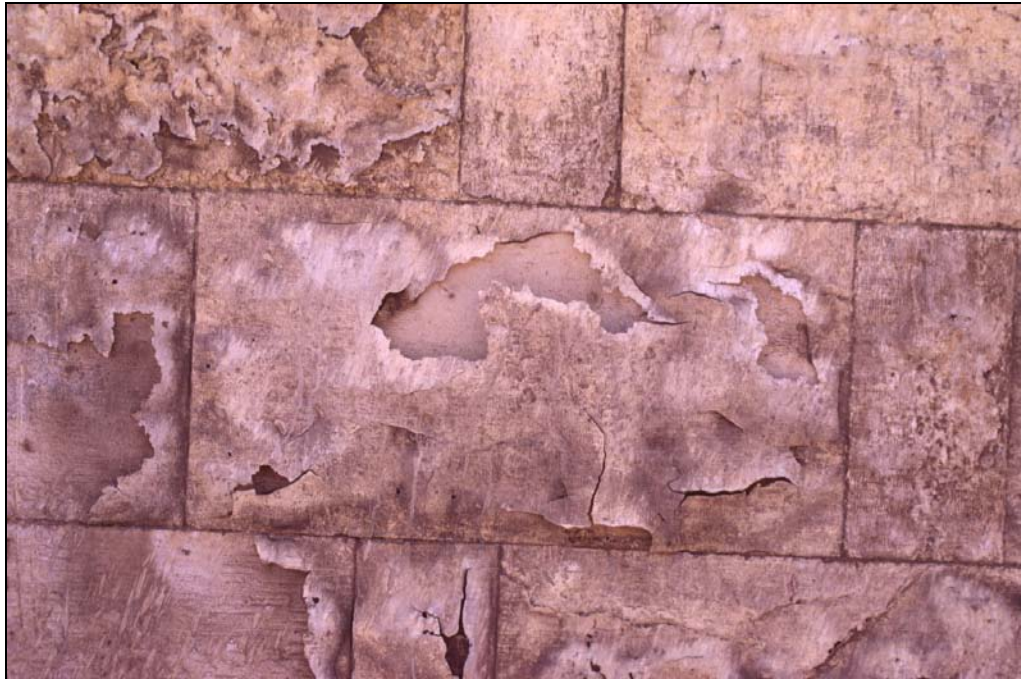
Figure IV.10 Detail of the thin salt crusts (veil) falling off in large plaques from the surface of the stones, 2000.
