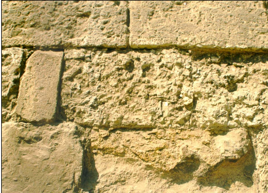
Figure I.11 Differential weathering of the veneer stones of the city wall.
