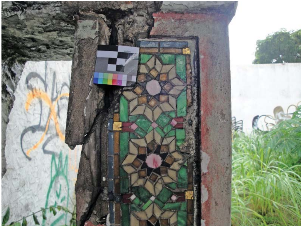
Figure 23: Rebar damage to porta-cochere column (source: by author, January,2010.)
