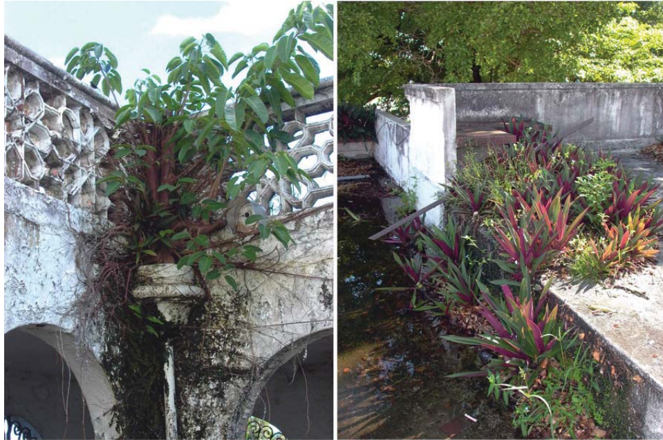
Figure 14: Villa Caparra clogged drains and plant growth on roof surfaces. (source: by Beatriz del Cueto, FAIA, 2010.)
