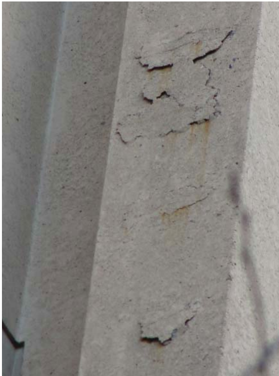
Figure 5.25- Cracks that can develop into spalls.
