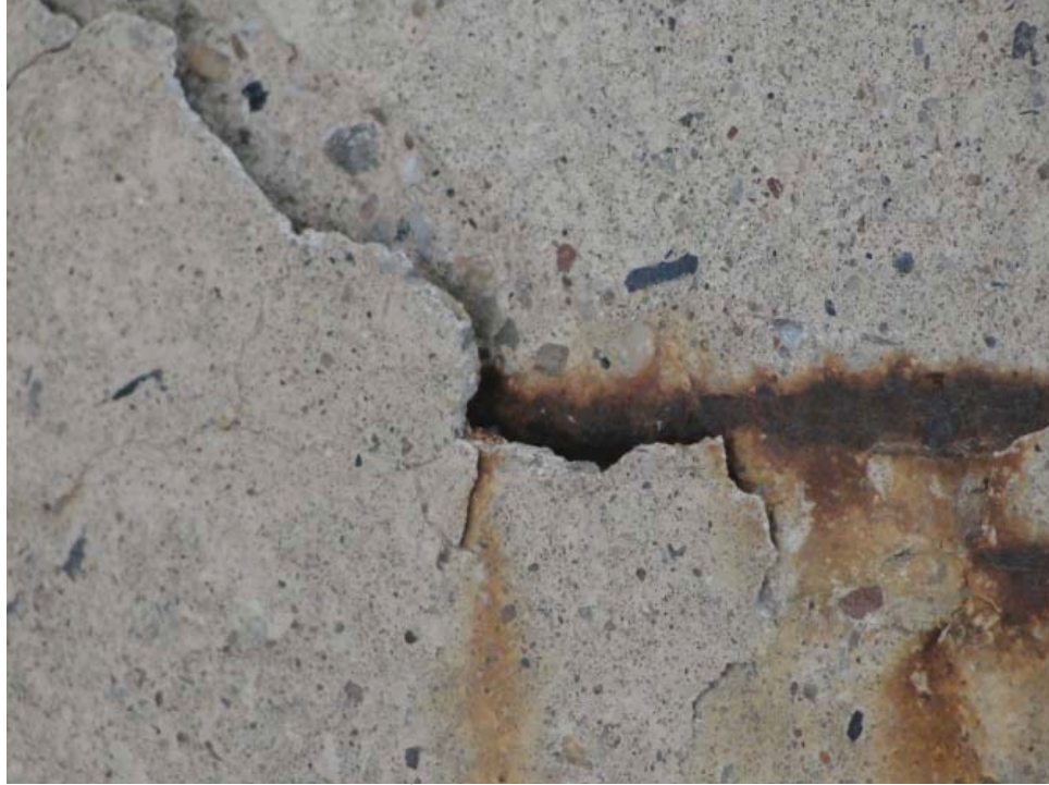
Figure 5.28- Spall on a column flange.
