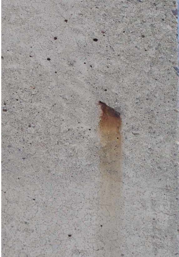
Figure 5.24- Corrosion stain associated with exposed reinforcement.
