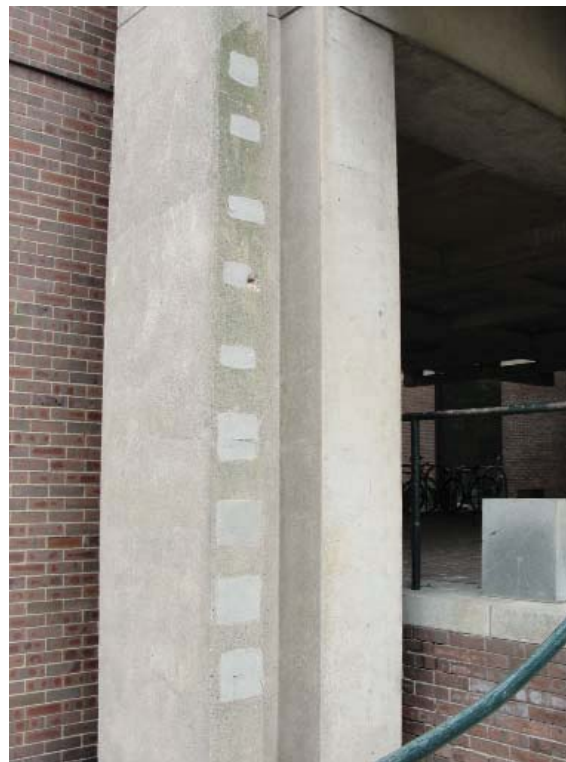
Figure 5.33- Patches on the ground floor level section of the northwest column on the north façade of tower.
