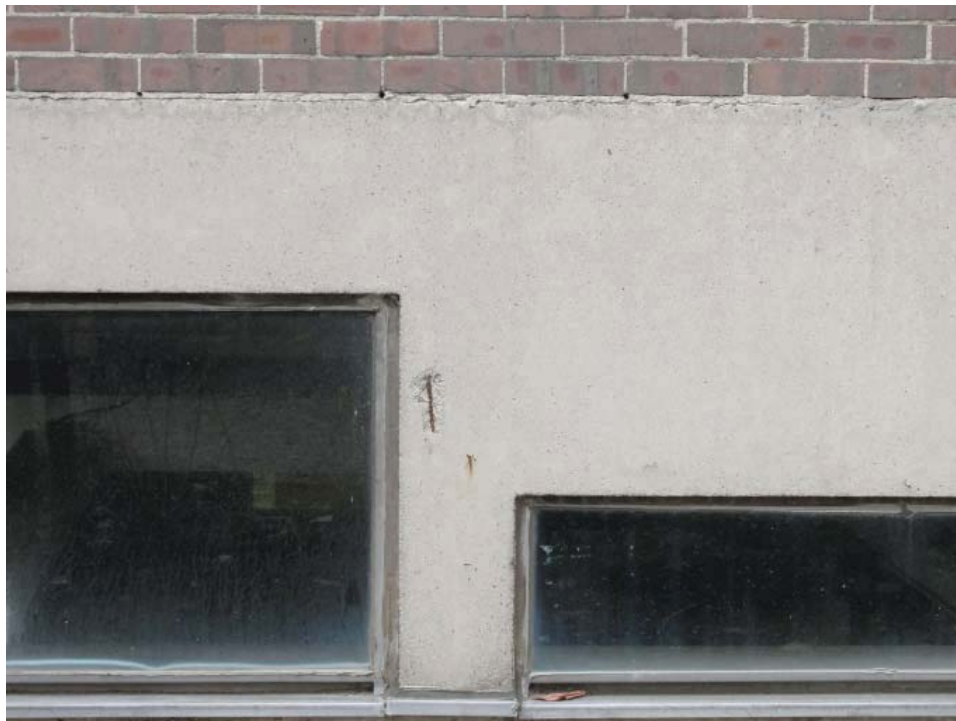
Figure 5.31- Exposed reinforcement on edge beam.
