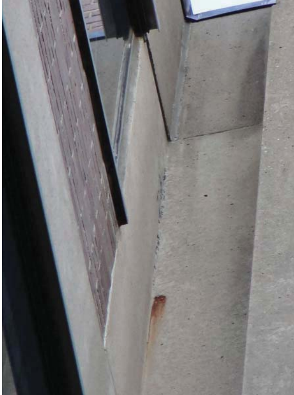
Figure 5.30- Exposed reinforcement, originally lacking concrete cover.
