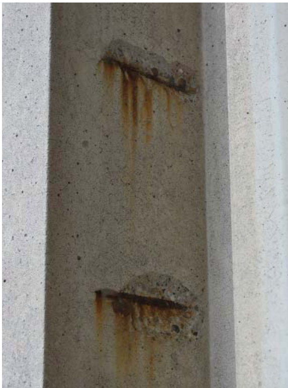
Figure 5.23- Corrosion stain associated with spall.
