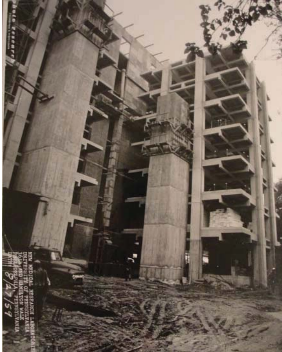
Figure 5.13- Construction photograph showing the cast-in-place structure of a subsidiary tower and the precast structure of a laboratory tower. (The Architectural Archive, University of Pennsylvania, 030.IV.A.490.12.45)
