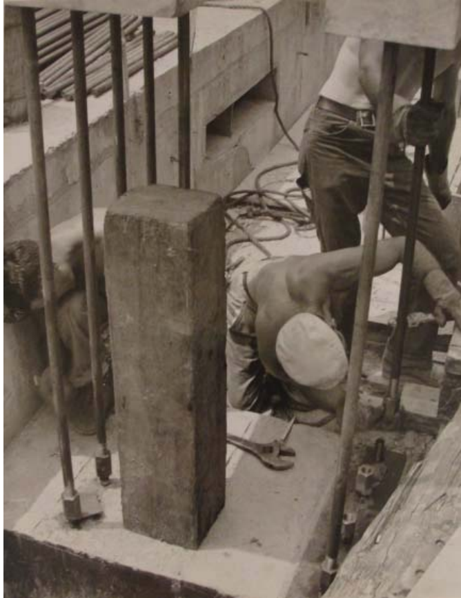
Figure 5.15- Column tendons being connected during erection of the pre-cast structure. (The Architectural Archive, University of Pennsylvania, 030. IV.A.490.11.1)
