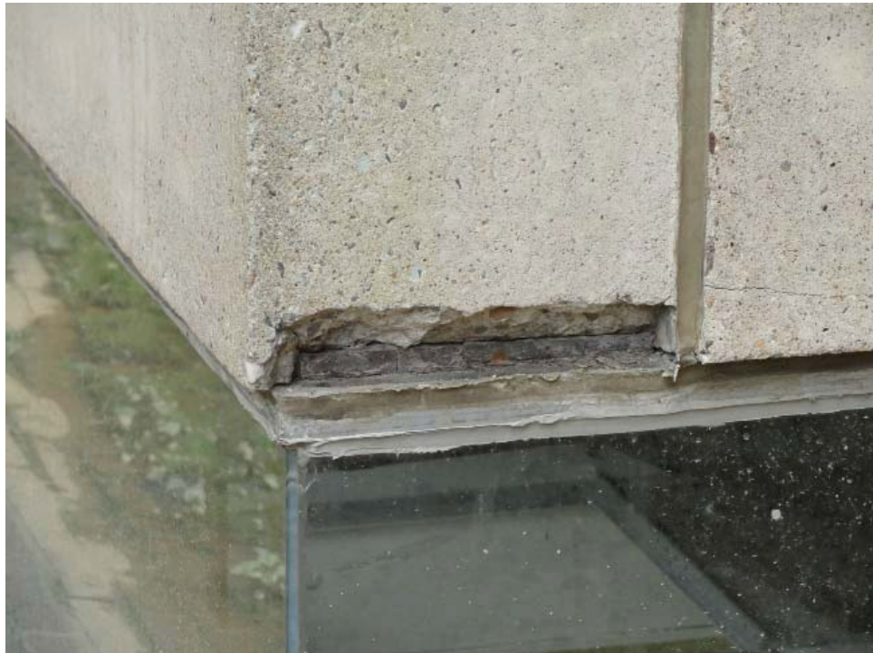
Figure 5.29- Spall on a window corner.
