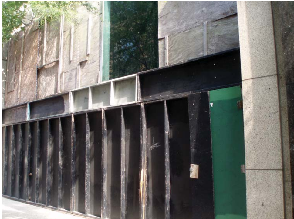
Figs. 5 and 6: These photos show the building, located at 1021 Chestnut Street and owned by Chestnut Associates, in July 2010. Its critically dilapidated condition is all the more alarming given its status on the Philadelphia Register, and reminds us that designation in no way covers the need to monitor. The failure to monitor in this case has effectively stripped a designated building of its significance.
