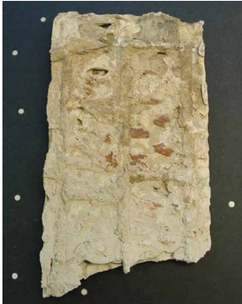
Figure 5.4. Backing of cornice segment that had fallen in May, 2008. Evidence of keying to the masonry is visible in the brick pattern imprint ( L. Vollono, 2009).
