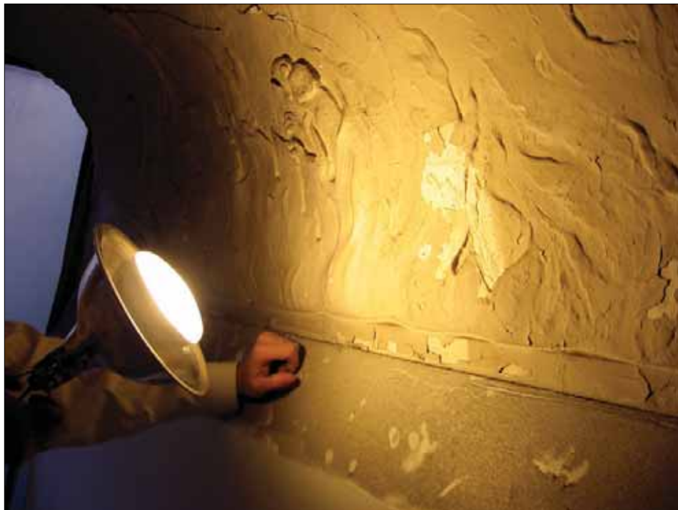
Figure 5.6. Curved cornice on East wall, with removed appliqué portion (GWAS2010.P2), November 2009. Old World chameleon figure is further evidence of applied pre-cast element, surrounded by a series of applied flames to visually and physically fix the element in place (L. Vollono, 2009).
