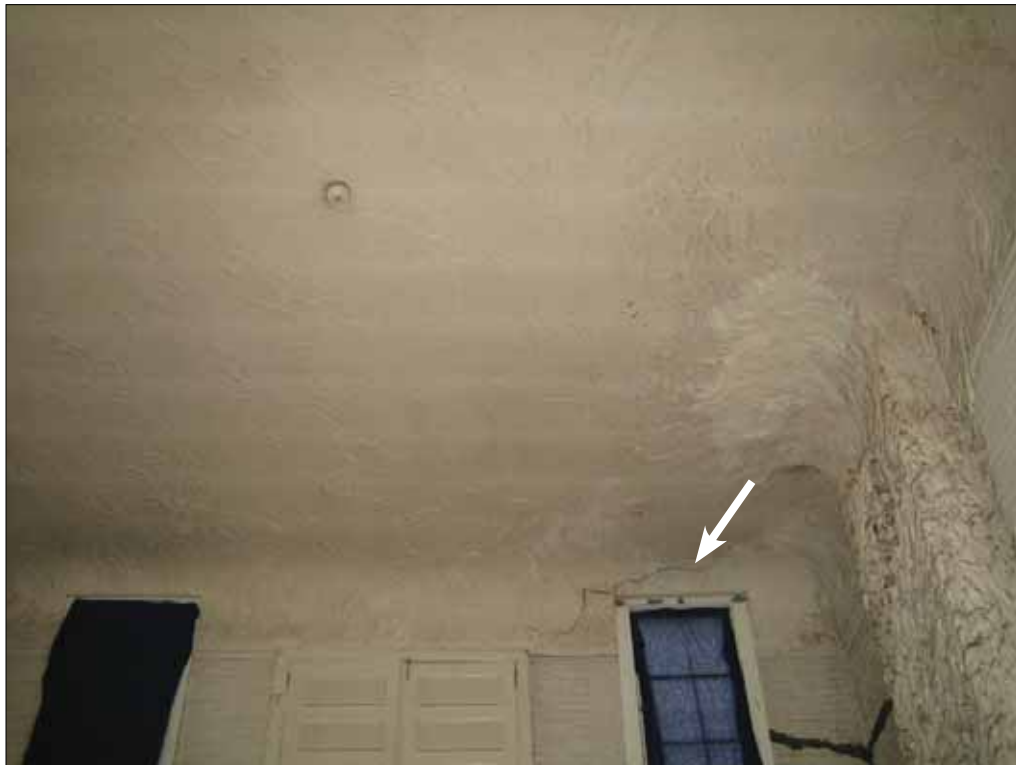
Figure 6.4. Ceiling cornice prior to cornice loss, November, 2006 (Archives of the New York Studio School).
