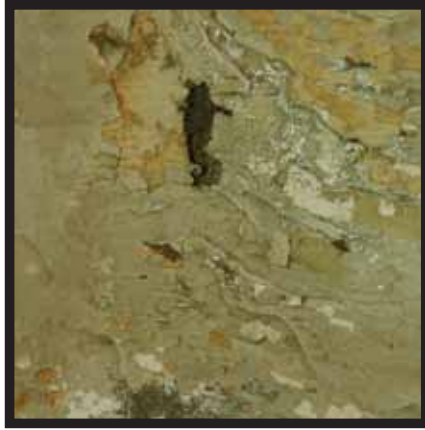
(a) plaster staining with wire mesh exposed
