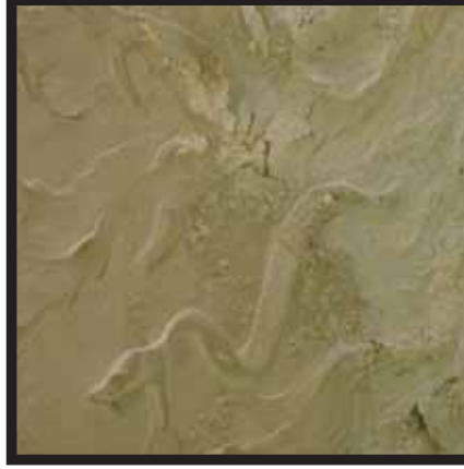
(c) loss due to extensive pitting
