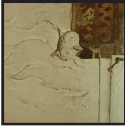
(a) cornice failure
