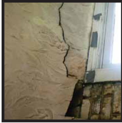
(a) abnormally large crack along cornice failure
