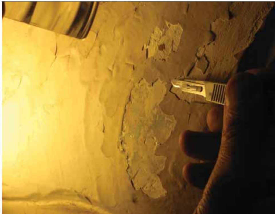
Figure 8.1. On-site paint exposure with a scalpel, conducted by Frank Matero (L. Vollono, 2009).
