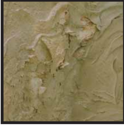
(b) vulnerable plaster due to paint loss
