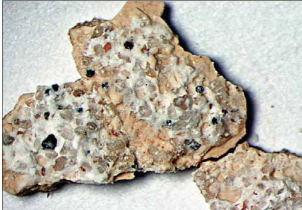
Figure 7.3. Macro photos of small detached sections of the paint that show the sandy finish plaster selectively attached to the back side of the gesso (J. Zucker, 2007).
