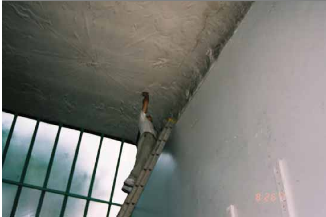
Figure 2.12. Brice Bowman (SuperStructures) measuring cracks in plaster, 2001 (Archives of the New York Studio School).
