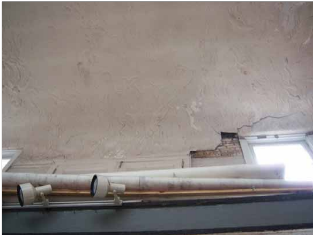
Figure 2.13. Following the cornice failure (L. Vollono, 2009).
