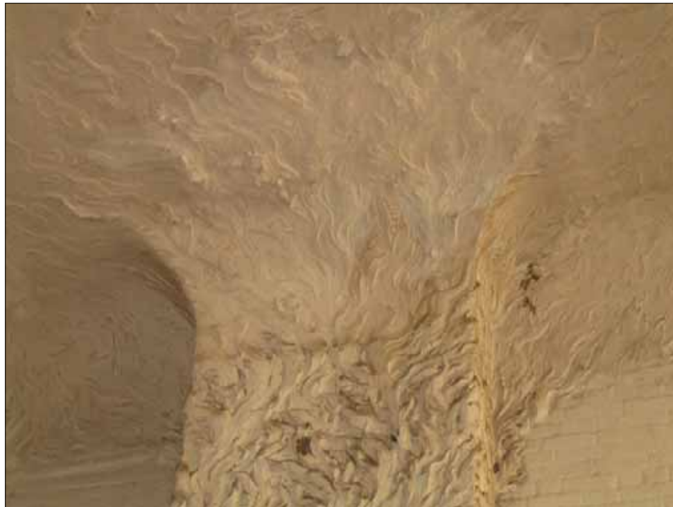
Figure 6.3. Detail of Pitting on Fireplace, 2006 (Archives of the New York Studio School).
