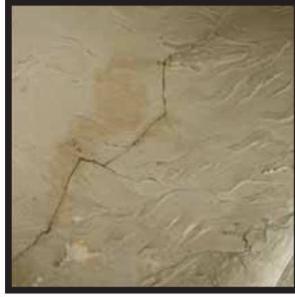
(c) staining due to prior treatment
