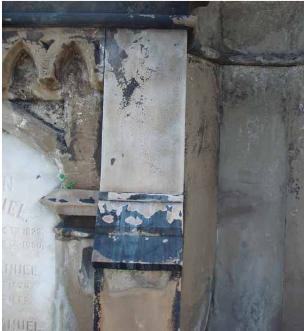
Figure 7.7 D/2 Solution did not remove soiling from case-hardened areas; note efflorescence post-cleaning (Source: E. Kemery, 2009)
