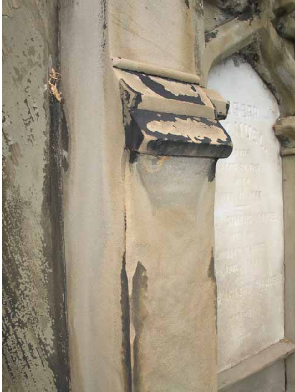
Figure 2.14 Pier of the Suddards-Manuel-Clark tomb with unique moulding feature (Source: E. Kemery, 2008)
