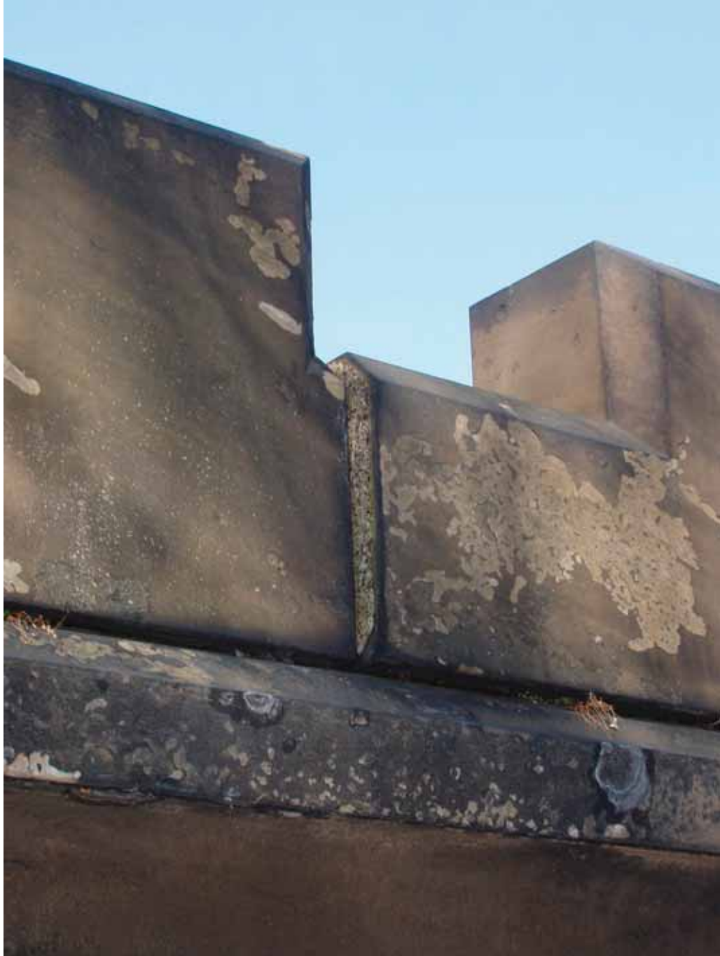
Figure 2.12 Recessed mortar joint on displaced crenellation (Source: E. Kemery, 2009)
