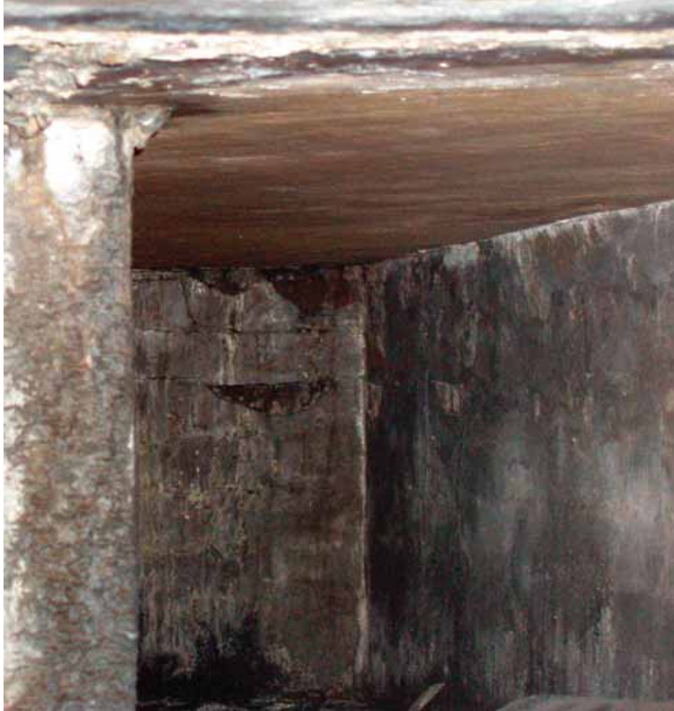
Figure 6.5 Interior of Suddards-Manuel-Clark vault showing efflorescence (Source: E. Kemery, 2009)
