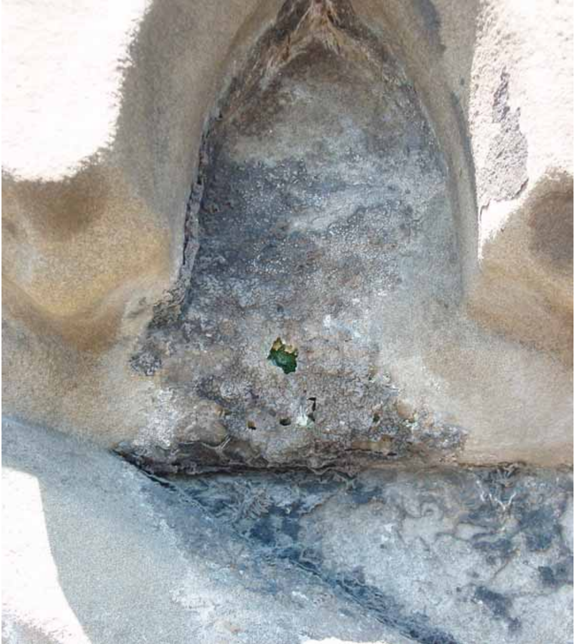
Figure 6.21 Microbiological colonization beneath blisters (Source: E. Kemery, 2009)
