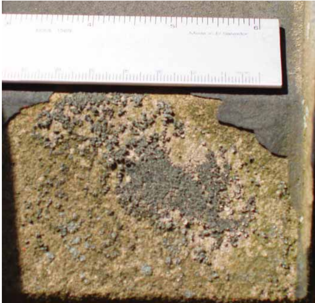
Figure 6.22 Microbiological colonization beneath peeling on crenellations (Source: E. Kemery, 2009)
