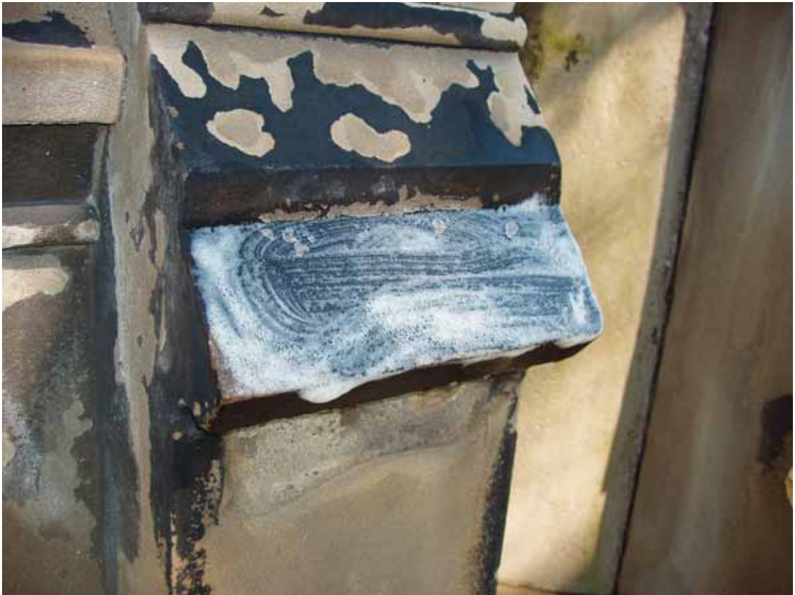
Figure 7.5 Section of opaque peeling/case-hardened crust during cleaning with Cathedral Stone® Products D/2 Biological Solution; D/2 Solution had no effect on case-hardened surfaces (Source: E. Kemery, 2009)
