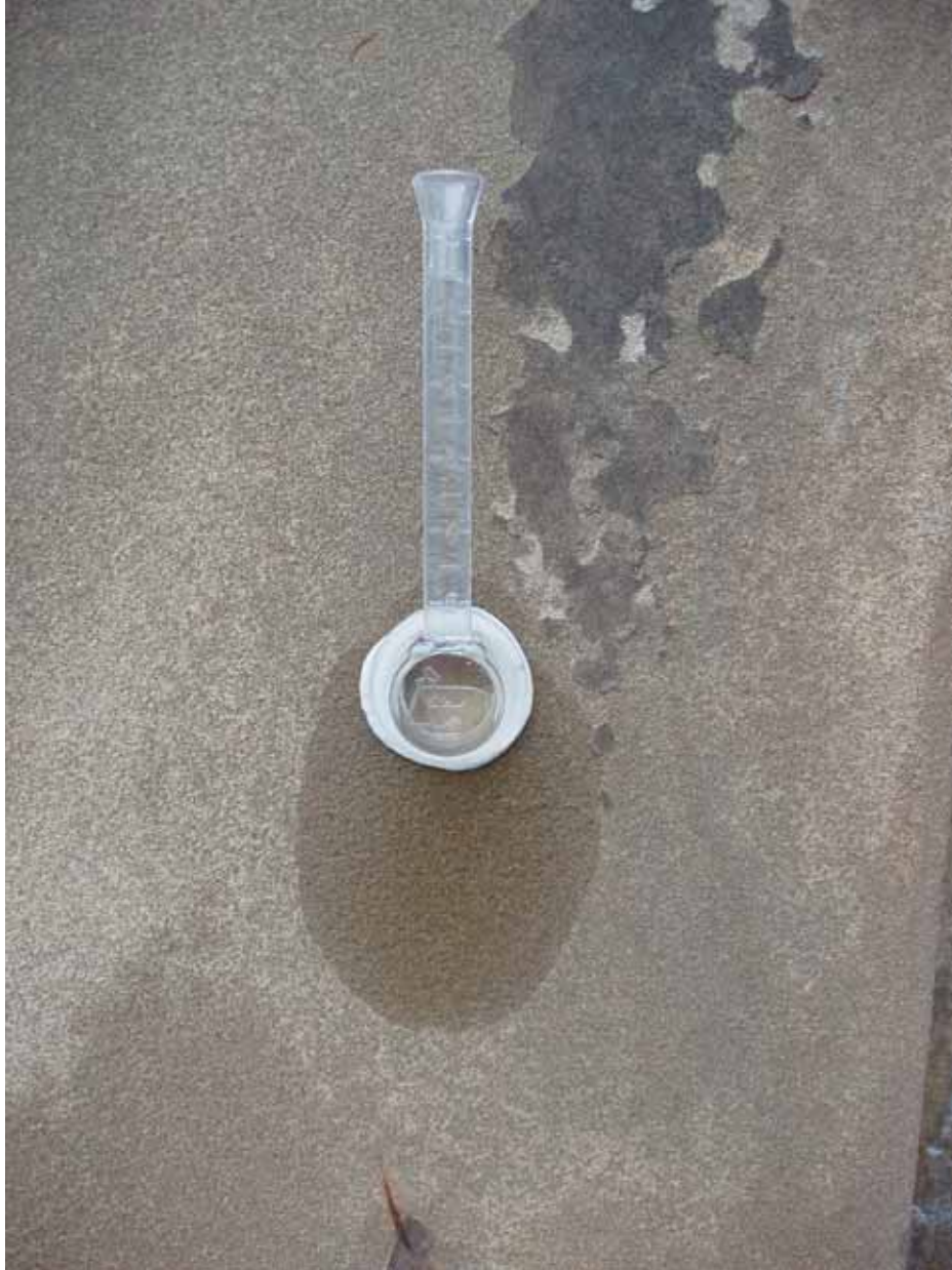
Figure 4.13 Failed RILEM tube testing in situ on a differentially eroded surface (Source: E. Kemery, 2009)
