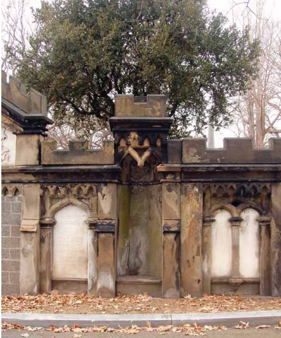
Figure 7.3 Section of the Suddards-Manuel-Clark monument to be cleaned, before cleaning with Cathedral Stone® Products D/2 Biological Solution (Source: E. Kemery, 2009)
