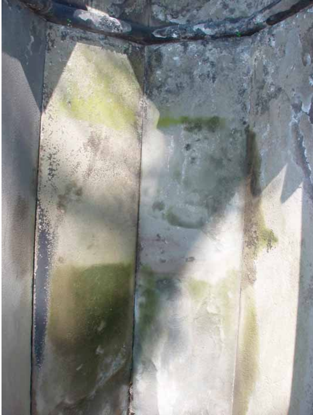
Figure 7.4 Cove after first cycle of Cathedral Stone® Products D/2 Biological Solution application (Source: E. Kemery, 2009)
