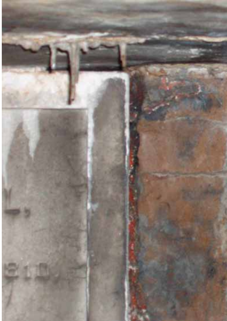
Figure 6.2 Interior of Suddards-Manuel-Clark vault showing brick sub-grade structure and white marble tablet (Source: E. Kemery, 2009)
