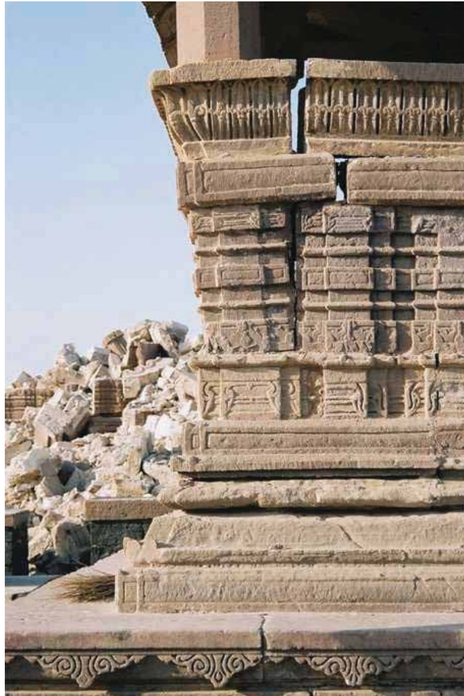
Figure 17. Vertical crack produced by seismic action. From www.conservationtech.com
