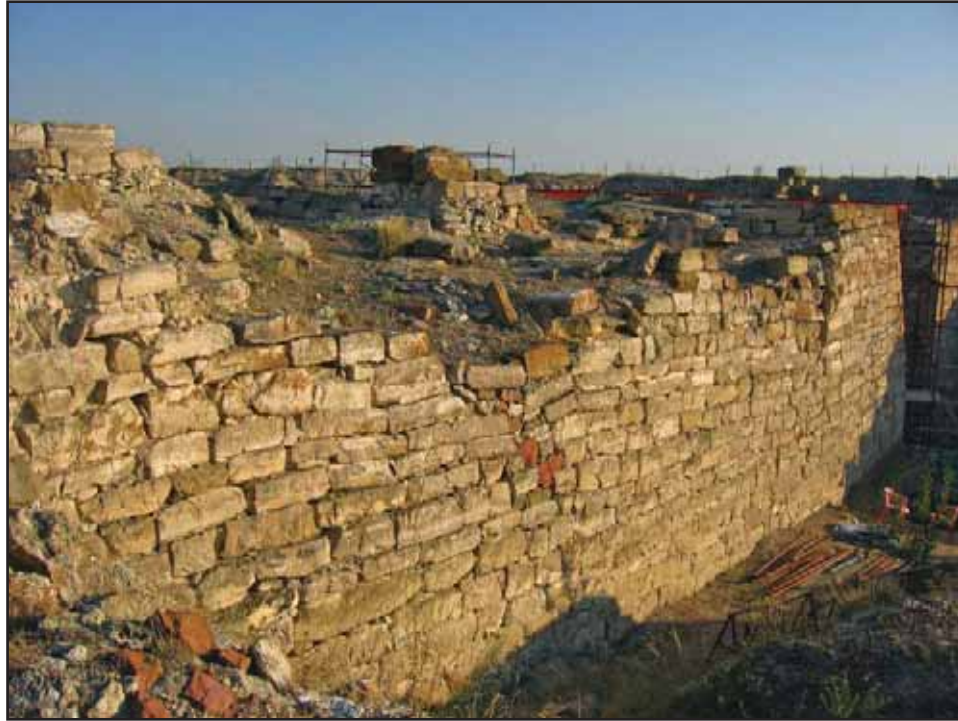
Figure 39. The general instability is evident in the South Court, which is only partially excavated. By Wong, 2006.
