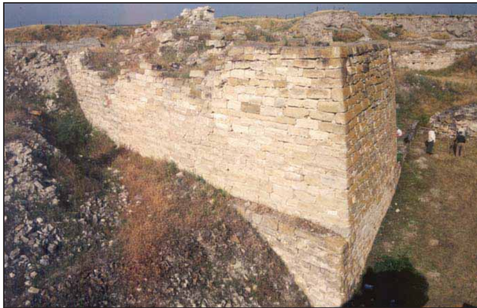
Figure 36. Displacements of the rubble core have increased the size of the bulge in the South Court wall. By Goodman, 2000.
