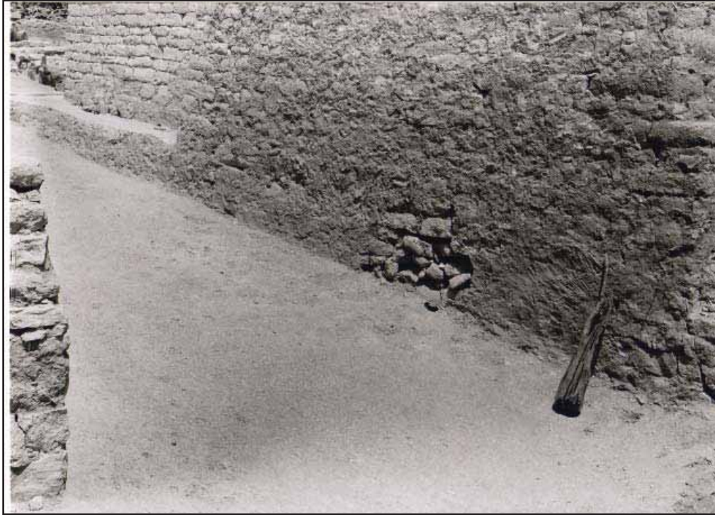
Figure 8. Extant earthen plaster on the southeast elevation of the North Court. From the Gordion Archives, ca. 1955.
