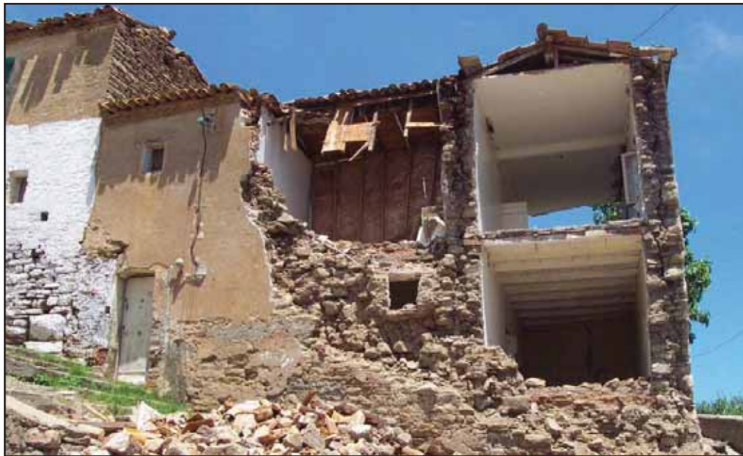
Figure 18. Failed corner of a multiple leaf system. From www.world-housing.net .
