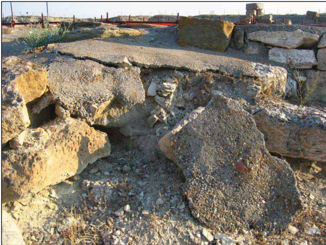
Figure 40. The concrete cap has failed in areas and allowed water to penetrate the core. By Wong, 2006.
