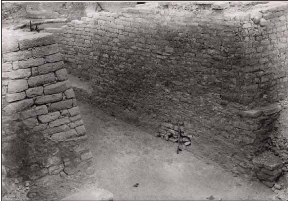
Figure 32. Southeast elevation of the North Court showing vertical cracks. From the Gordion Archives, ca. 1955.
