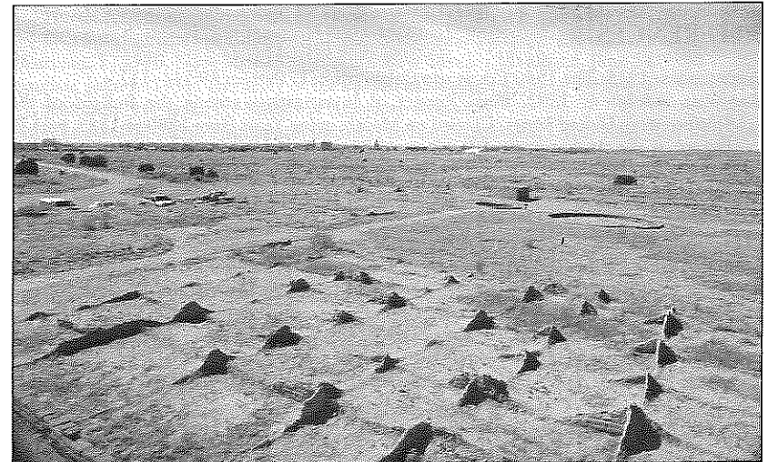
Figure 4.7 Wall erosion at Kuaua, 1997. (Photograph by Frank Matero.)
