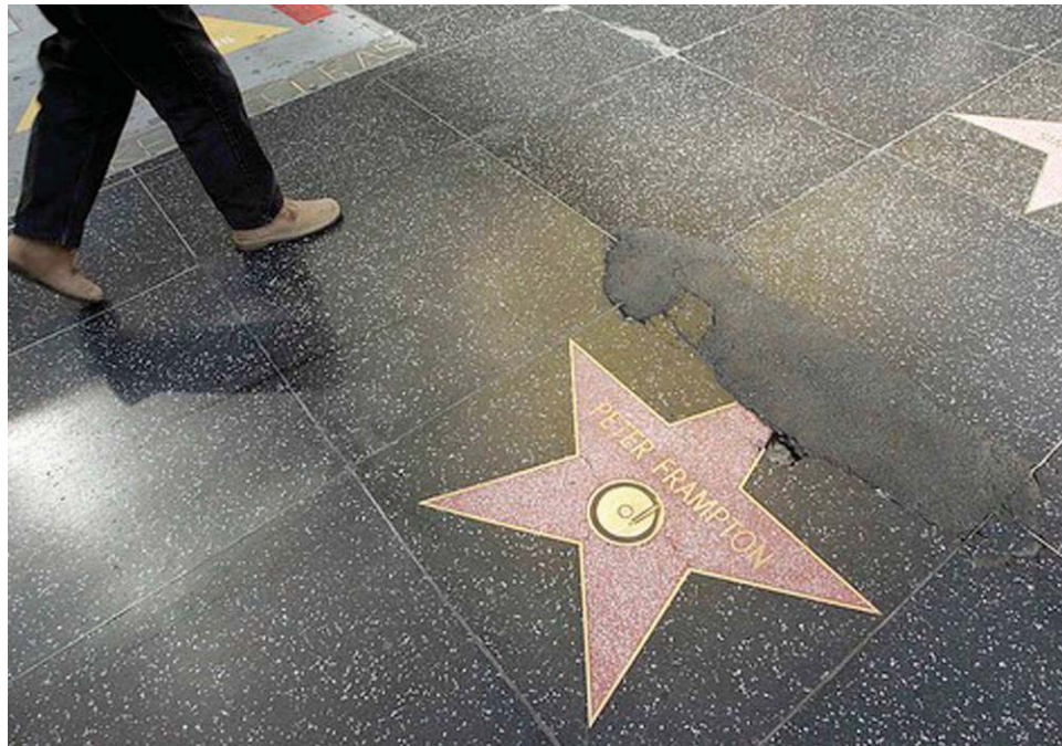
Figure 7: A damaged and patched terrazzo star from the Hollywood Walk of Fame. Source: Loss Angeles Times, February 9, 2007. http://www.latimes.com/news/local/la-me-stars9feb09,1,3826359.story?page=2&cset=true&ctrack=1&coll=la-headlines-california
