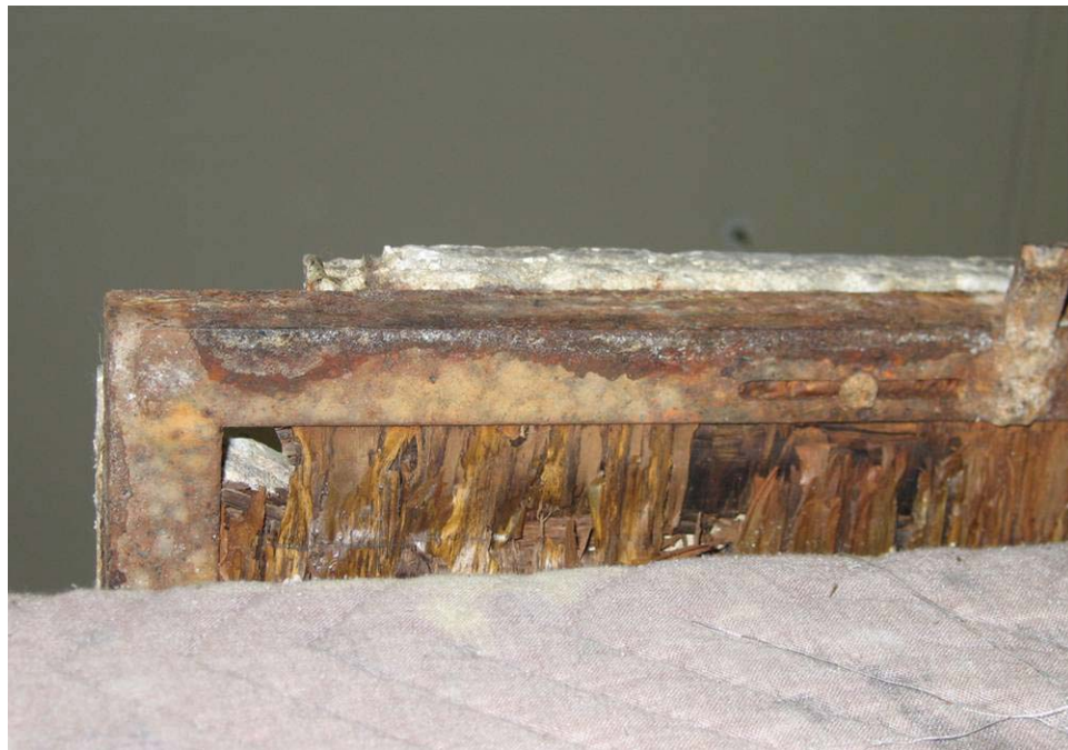
Figure 15: View of a terrazzo tile from below with rotting plywood. Source: Photo by author.
