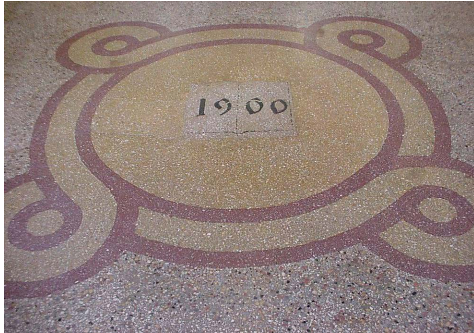
Figure 5: Before restoration of the terrazzo in St. Joseph's Library, St. Joseph Missouri. Source: http://www.ntma.com/07_2005_honor_awards_desc.php?job_name=stjoseph1
