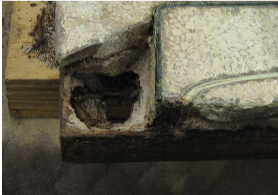
Figure 14: Detail of a damaged terrazzo tile showing the metal frame, terrazzo, underbed and a hold where the plywood support has rotted. Source: Photo by author.
