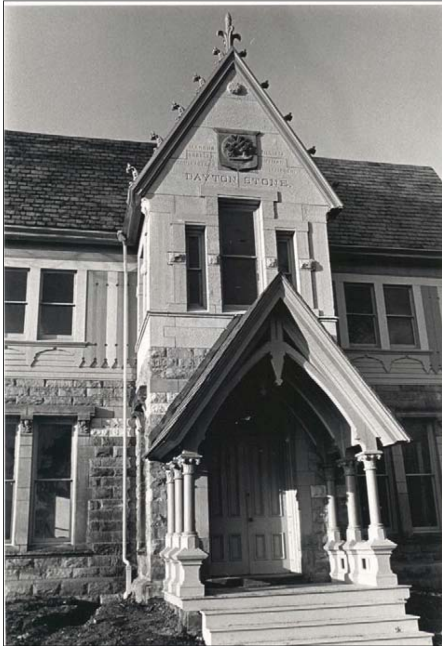
Figure 1.4: South elevation of Ohio House after Bicentennial restoration efforts 1976, note absence of pyrite staining in “DAYTON STONE” limestone in projection gable (Fairmount Park Commission.).
