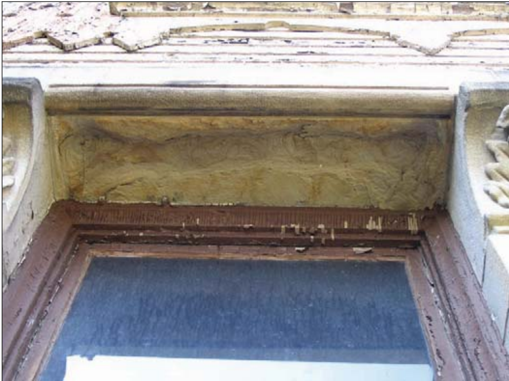
Figure 5.2: Detail of underside of window lintel on south façade, stone displays over 2 inches of loss.
