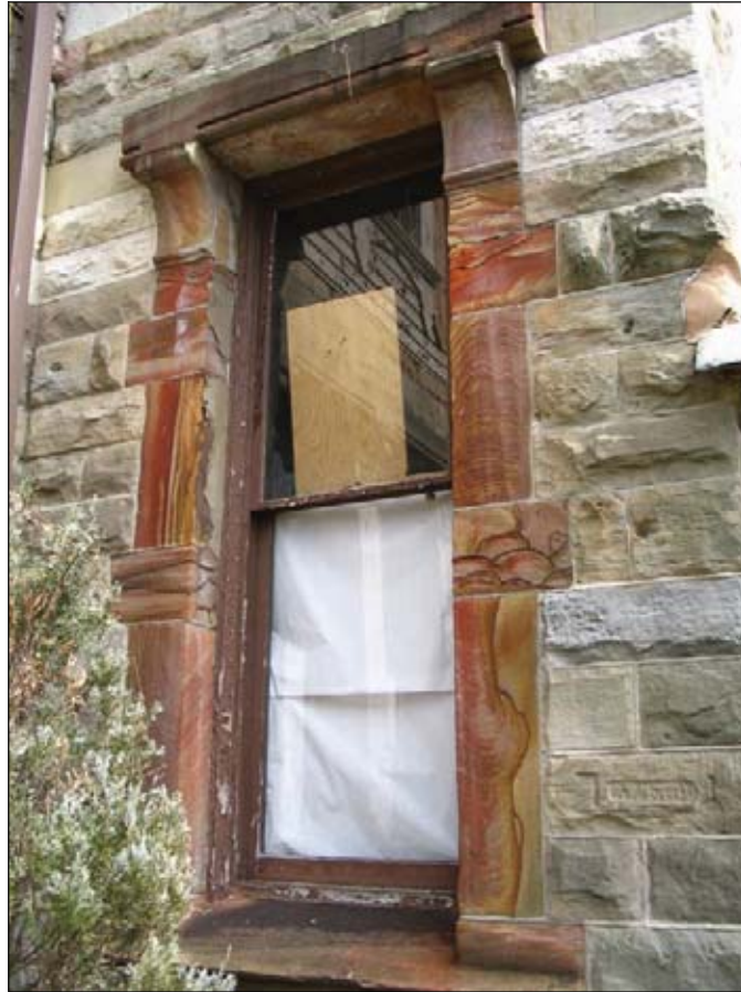
Figure 3.1: Liesegang rings in sandstone in window surrounds in front bay.
