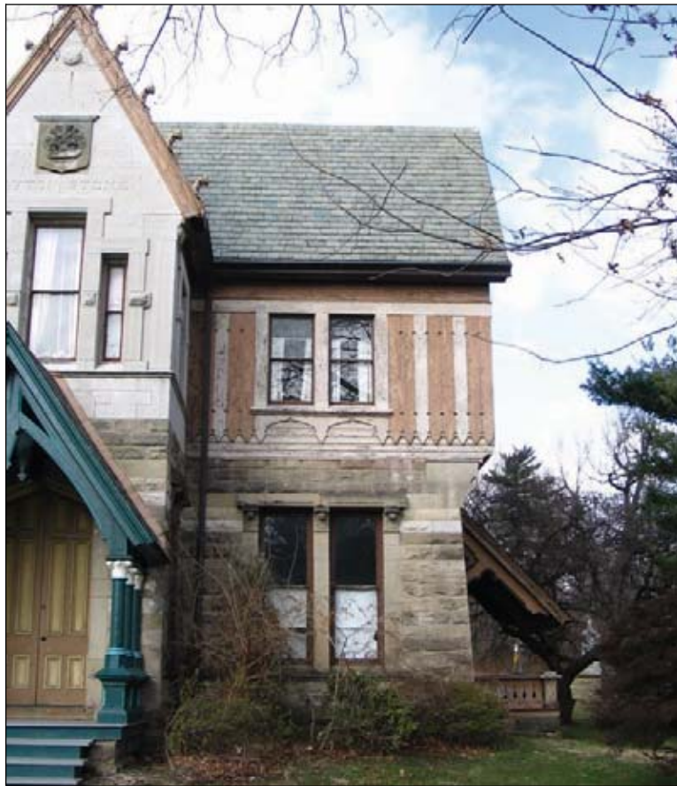
Figure 5.5: Photo illustrating proximity of shrubbery to deteriorated area of lower right side of south façade.
