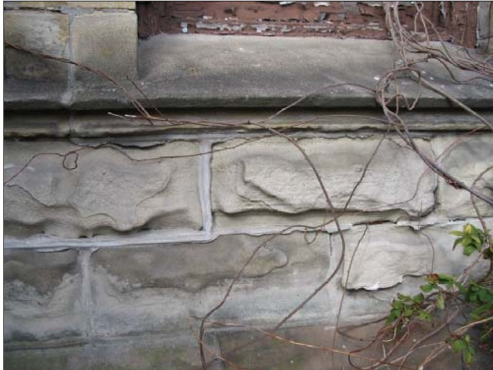
Figure 5.6: Detail of deteriorated area of lower right side of south façade due to stronger summer sun exposure.
