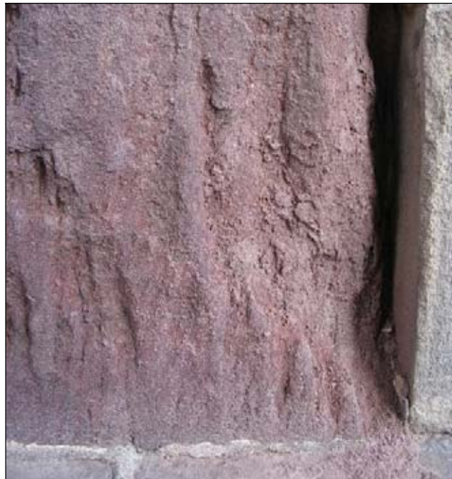
Figure 5.4: Detail of deteriorated of lower right stone in the Coshocton sandstone (Coshocton & Co) window surround.
