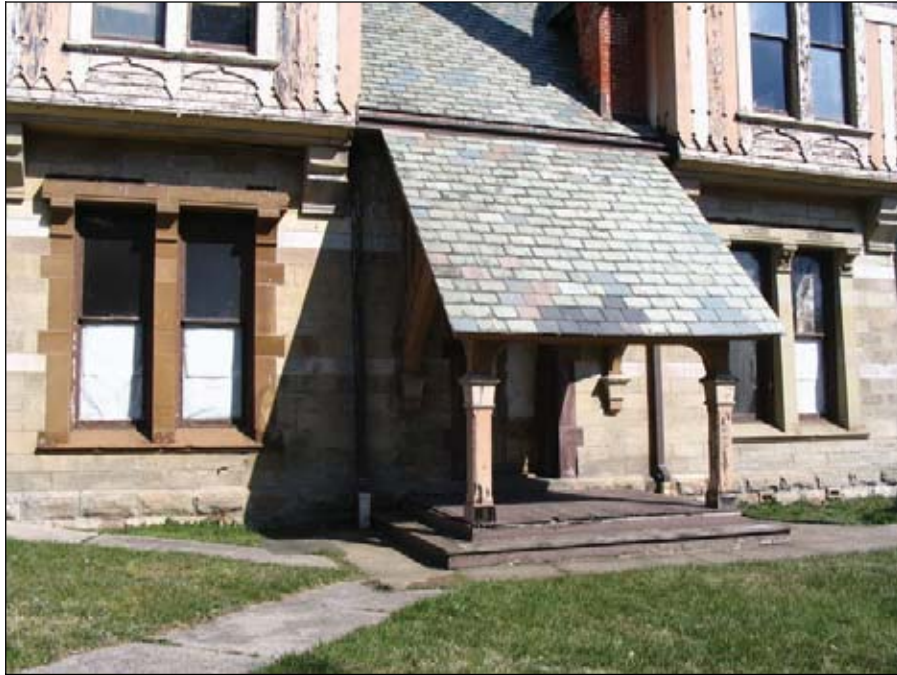
Figure 5.3: Photo illustrating path of strong sun exposure on west façade and areas of shade from the porch, note the exposure of lower right stone in the Coshocton sandstone (Coshocton & Co).
