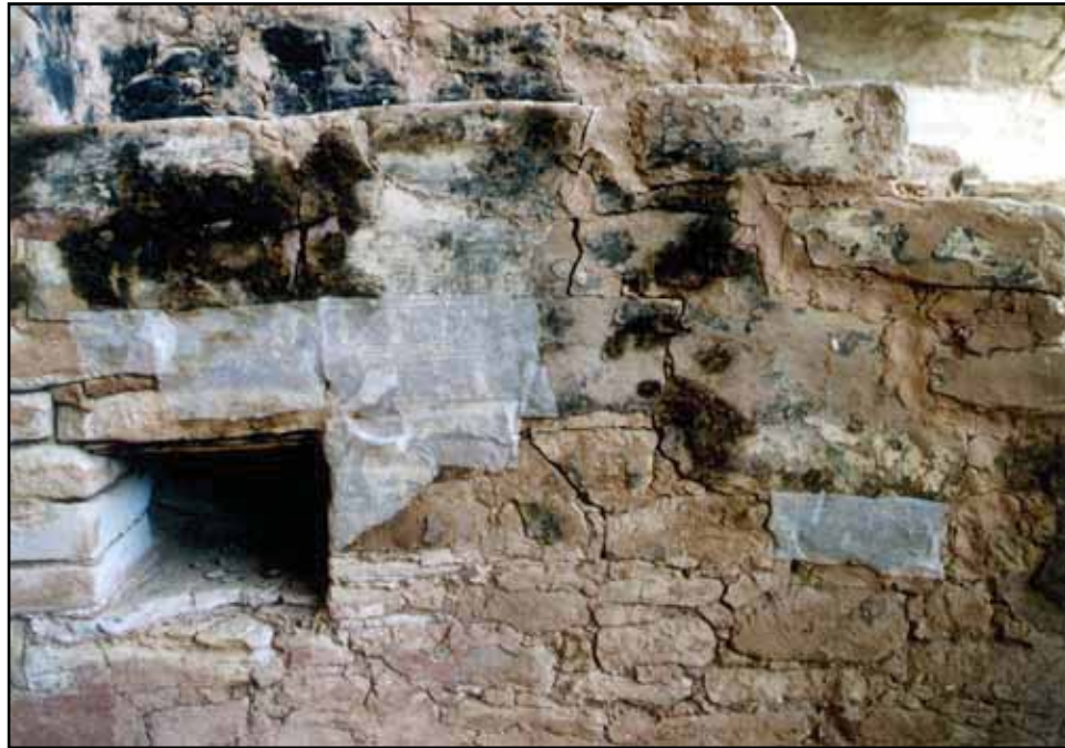
Figure A.22. Japanese facing paper in place as an emergency plaster conservation treatment (Fiero 11/04/1994).
