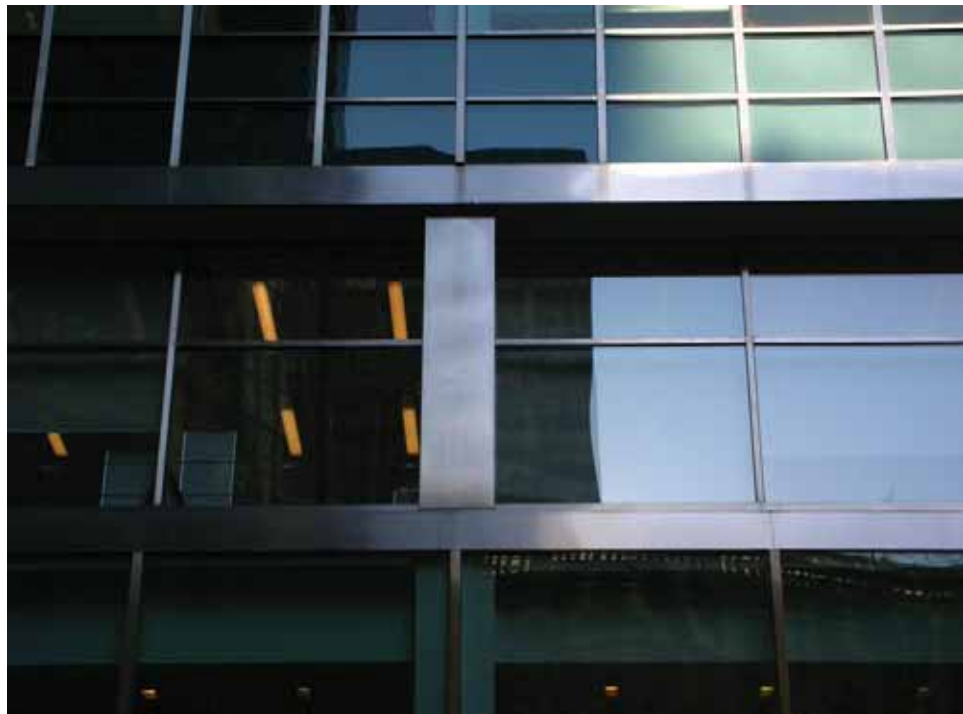
Figure 6.4 - Lever House curtain wall after replacement, view from interior courtyard, photo by E. Buckley 19 Dec. 2006.
