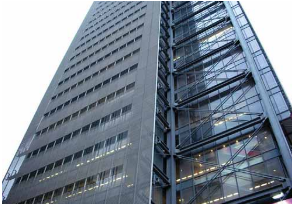
Figure 8.2 - Shaft of New York Times Tower under construction, photo by E. Buckley 19 Dec. 2006.
