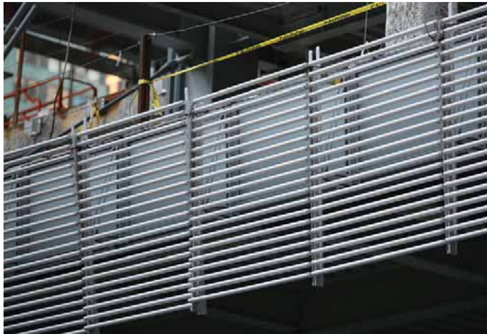
Figure 8.4 - New York Times Tower - network of ceramic tubes under construction, photo by E. Buckley 19 Dec. 2006.
