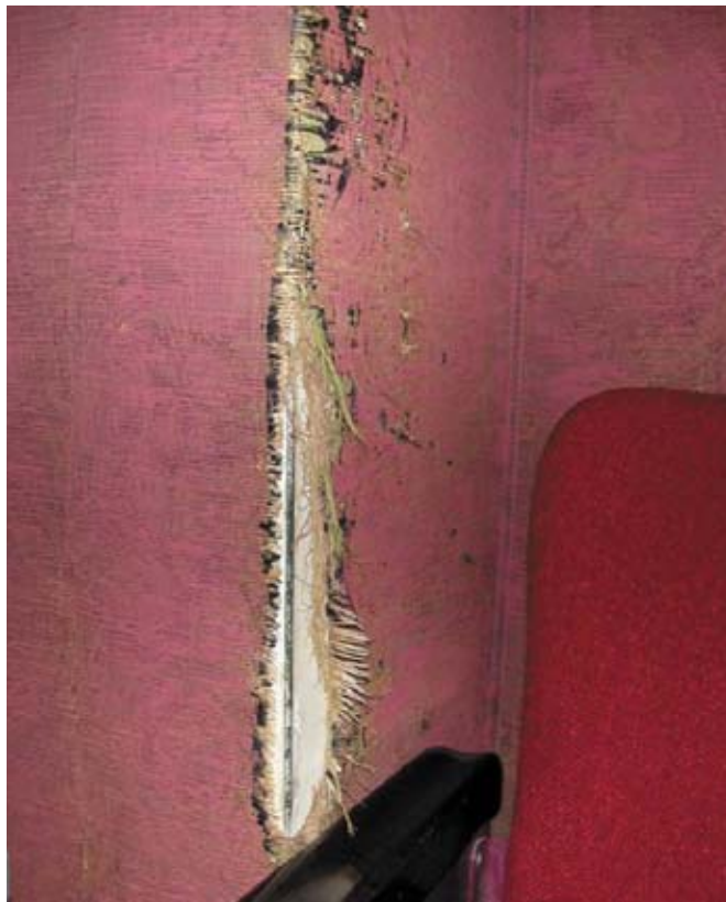
Fig. 46, Above , Fabric Pulling Away from Wall
