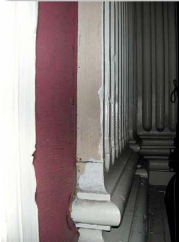
Fig. 32, Above , Pilaster Base with Chipped Paint
