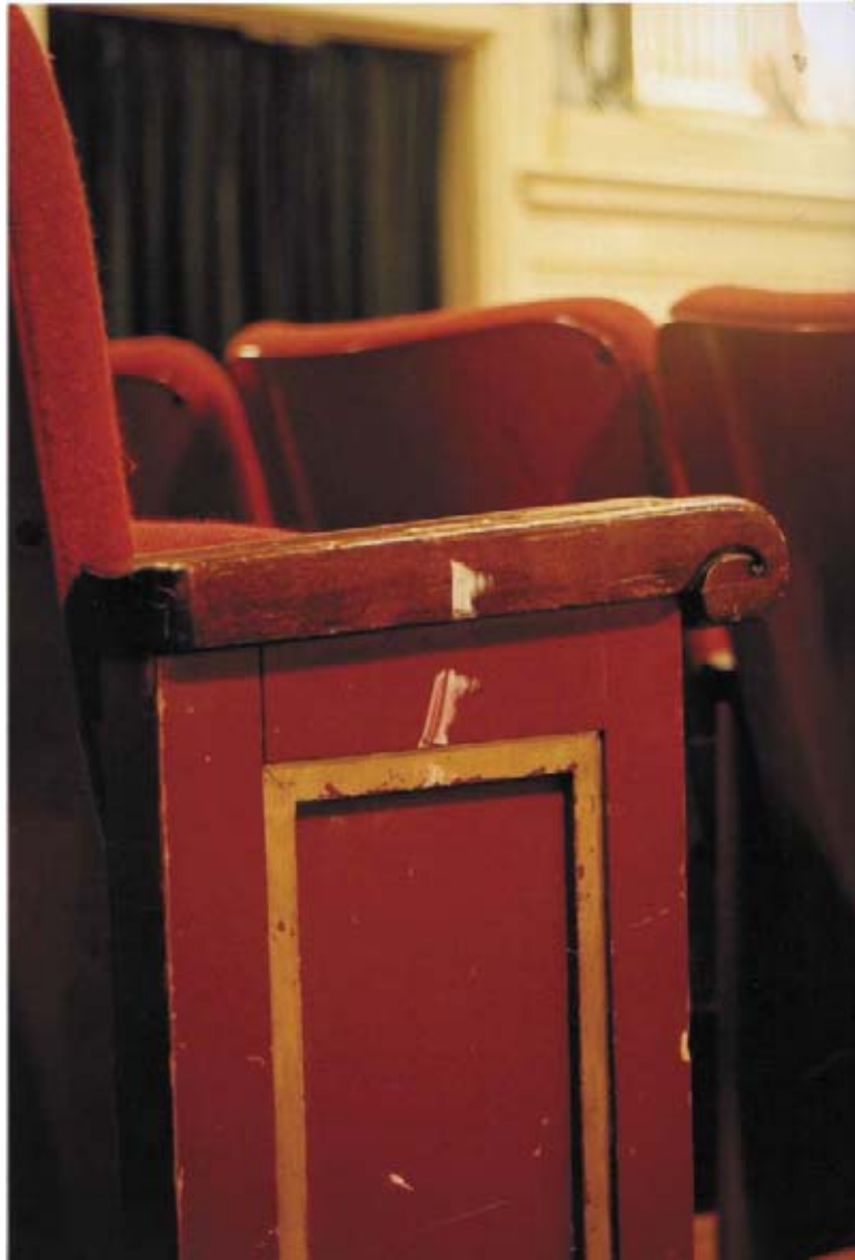
Fig. 31, Auditorium Stanchions with Red and Gold Paint and White Paint Drips
