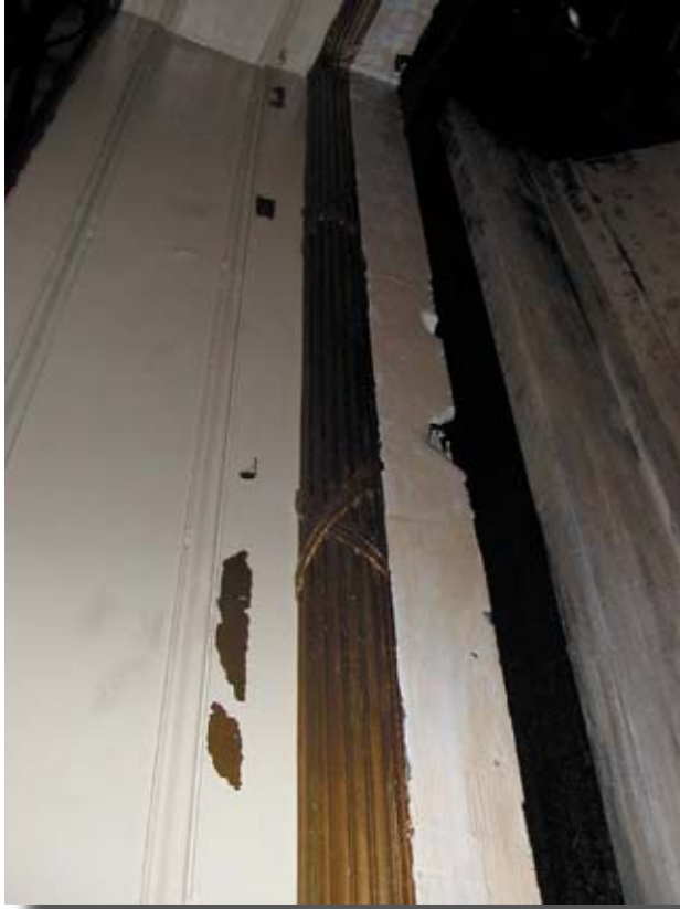
Fig. 37, Left , Damage to Proscenium
