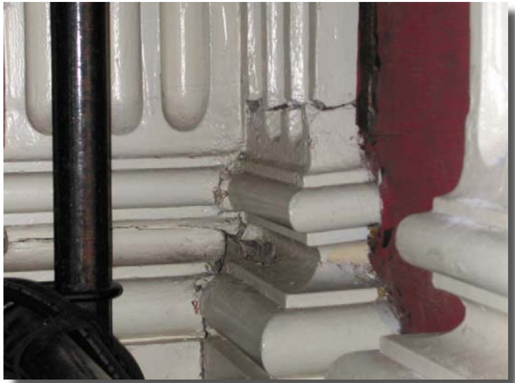
Fig. 39, Horizontal Cracking at Pilaster Bases
