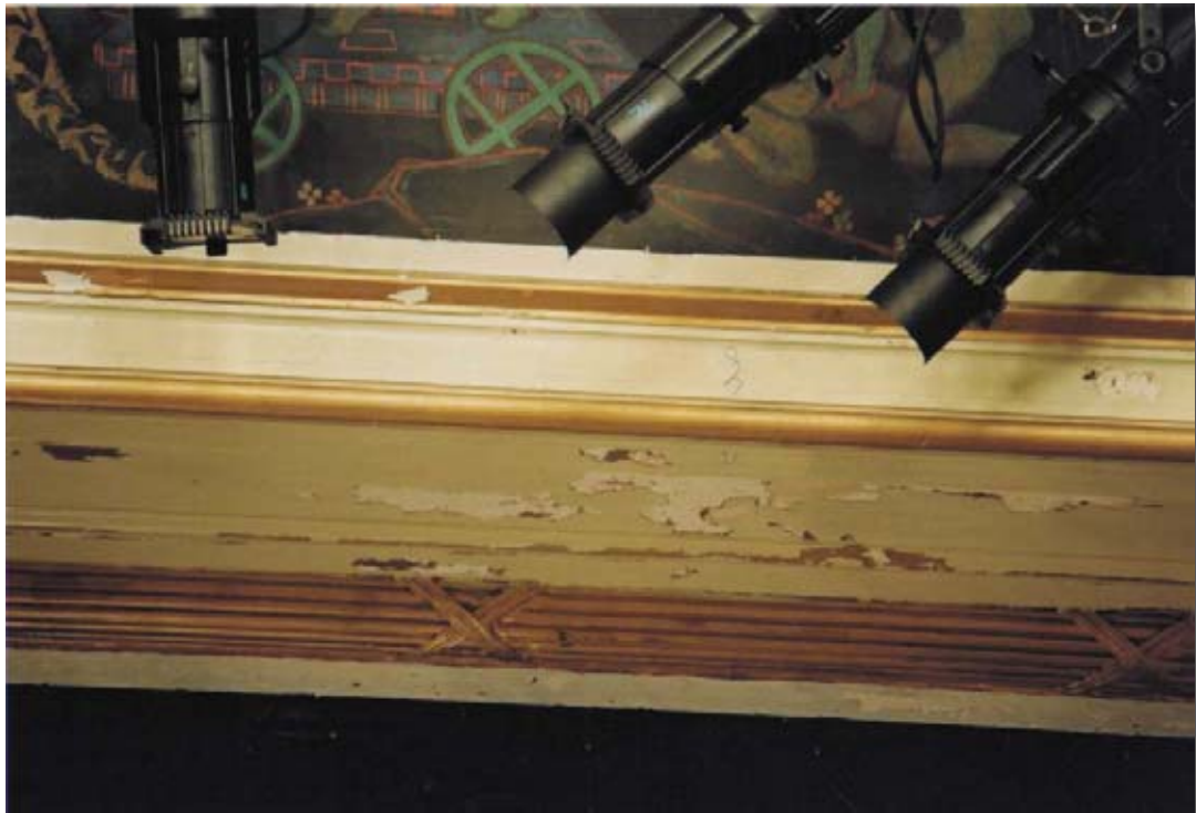
Fig. 36, Chipping Paint on the Proscenium
