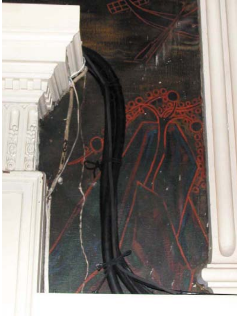
Fig. 57, Cables Run Through House, Obstructing Mural and Putting Weight on Moulding
