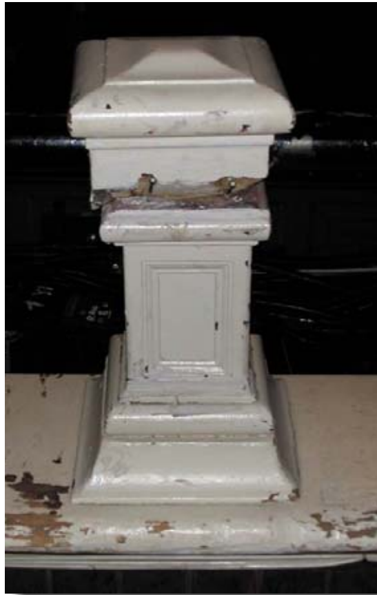
Fig. 41, Left , Damaged Balcony Post
