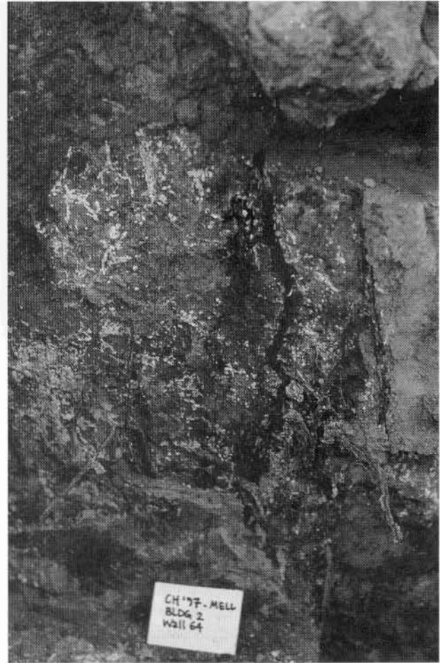
Figure 6.1. South area, Building 2/Wall 64. Wall plaster detachment and collapse from root growth, salts, and desiccation during excavation. (Photo: F. Matero.)
