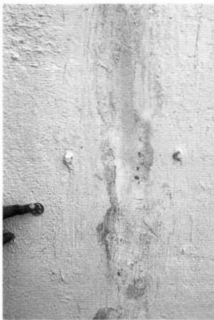
Fig. 2. Surface damage resulting from expansion cracks and subsequent repairs and repainting on the rotunda's concrete skin, 1996. Courtesy of the University of Pennsylvania's Architectural Conservation Laboratory.
