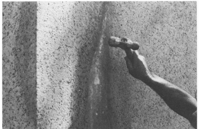
18. Ineffective hand removal of deposits.
