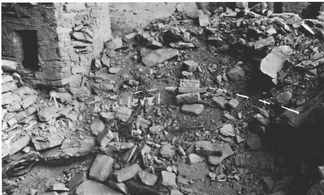
Fig. 9. Kiva C. Mug House, 1935, before repair. Courtesy of NPS-MEVE
