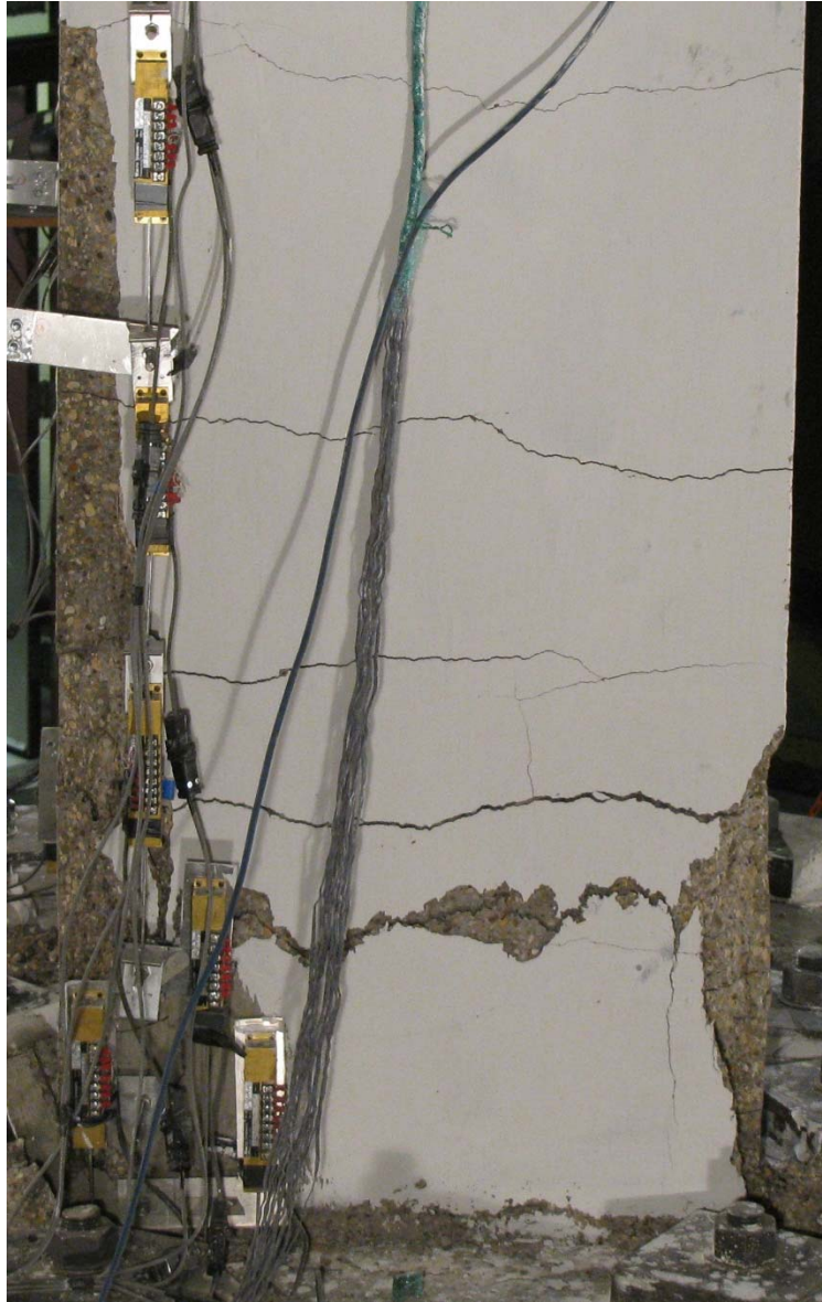
Figure 5.27. Observed Damage at the Beginning of “Moderate” Damage Category
