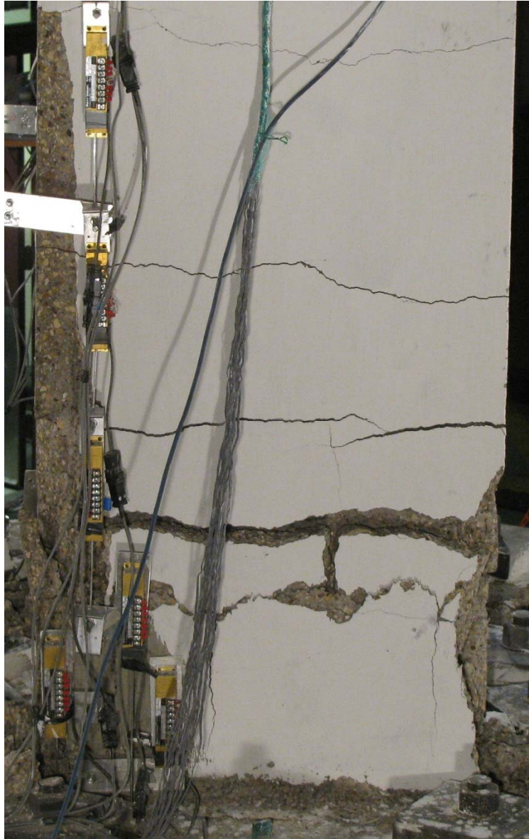
Figure 5.28. Observed Damage at the Beginning of “Severe” Damage Category
