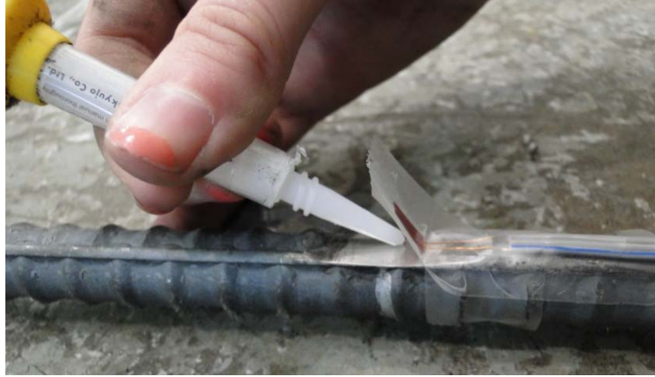
Figure A.8. Attaching the Strain Gage to the Prepared Surface of the Bar
