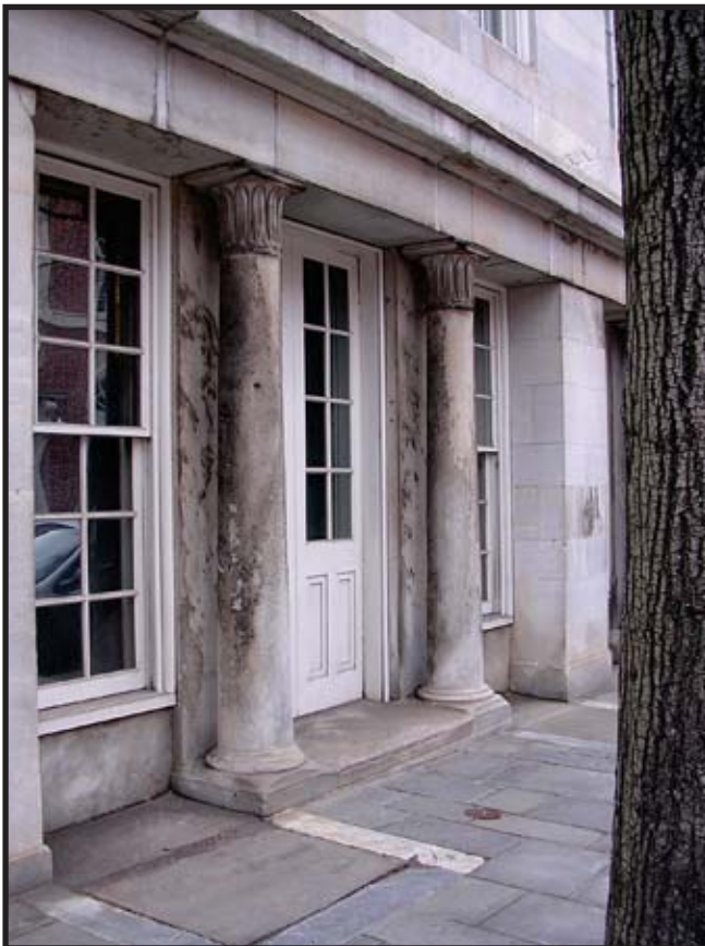
Figure C.51: South elevation, columns 3 and 4 Source: University of Pennsylvania South wall, second entrance from west end. Date: Winter 2005
