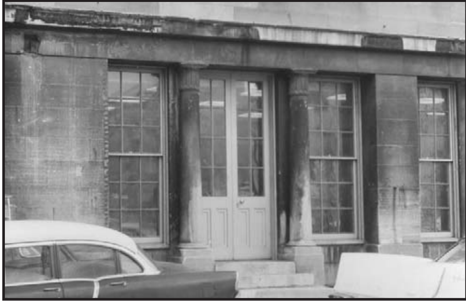
Figure C.21: North elevation, columns 3 and 4 (second bay from the east) Source: INHP Archives Caption: Merchants' Exchange – bay deterioration Creator: W. A. McCullough Date: March 16, 1961
