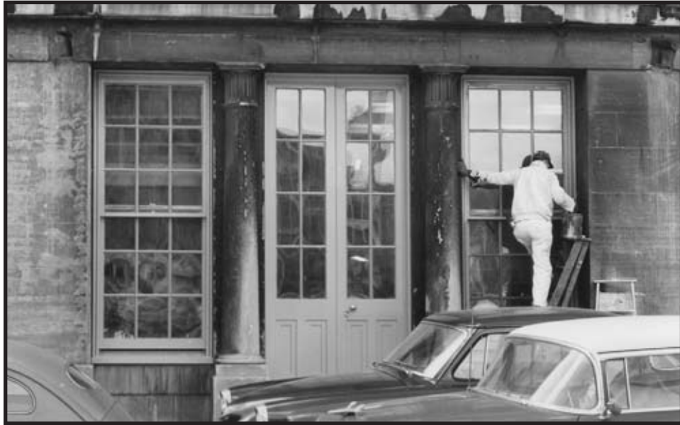
Figure C.23: North elevation, columns 1 and 2 (first bay from the east) Source: INHP Archives Caption: Merchants' Exchange – bay deterioration Creator: W. A. McCullough Date: March 16, 1961
