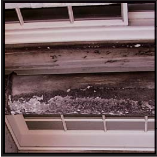
(a) blistering in areas of flaking and contour scaling
