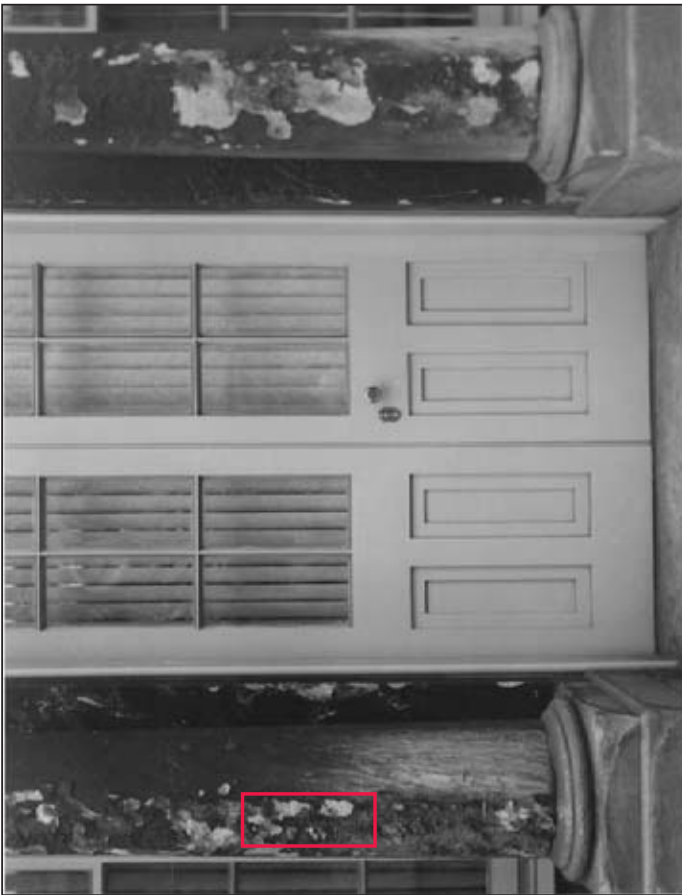
Figure 4.18: South Elevation, columns 9 and 10 Source: INHP Archives Caption: Merchants' Exchange marble deterioration Creator: W. A. McCullough Date: April 5, 1961
