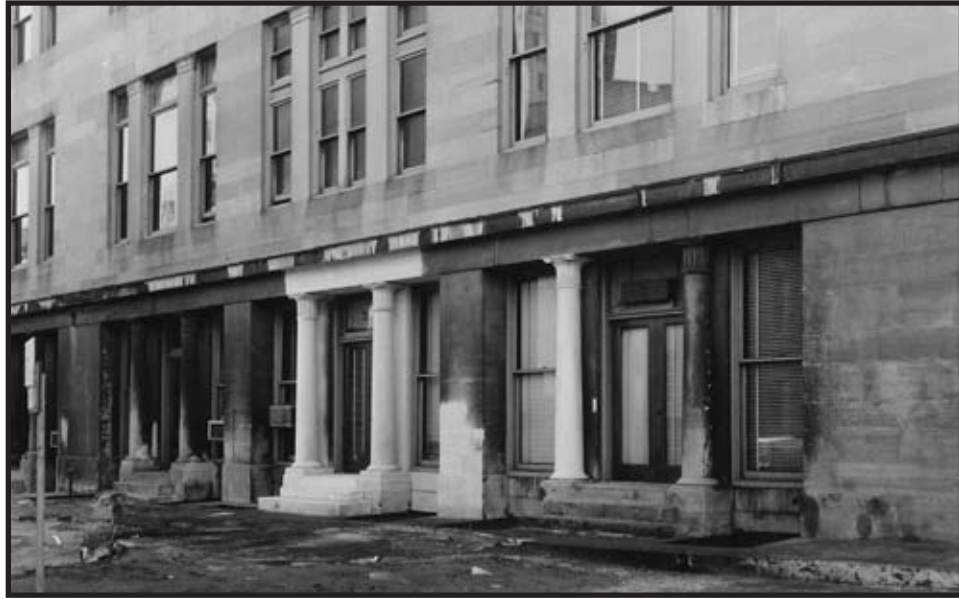
Figure C.17: North elevation, columns 6-10 Source: INHP Archives Caption: Merchants' Exchange: 2 columns treated by sandblasting and 1 column carved by stone cutter Creator: Paul J. F. Schumacher Date: December 15, 1953
