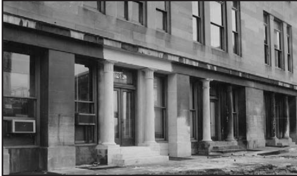
Figure C.15: North elevation, columns 5-10 Source: INHP Archives Caption: Merchants' Exchange: 2 columns treated by sandblasting and 1 column carved by stone cutter Creator: Paul J. F. Schumacher Date: December 2, 1953
