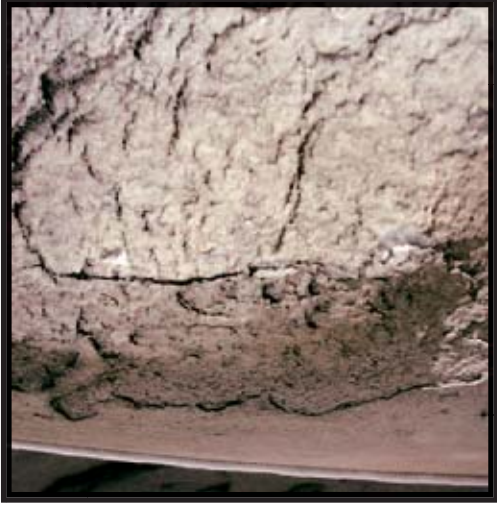
large blister detaching from stone surface
