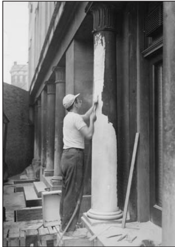
Figure 2.7: Merchants’ Exchange: Re-carving of North elevation column by Milione, May 1953. From the INHP Archives.
