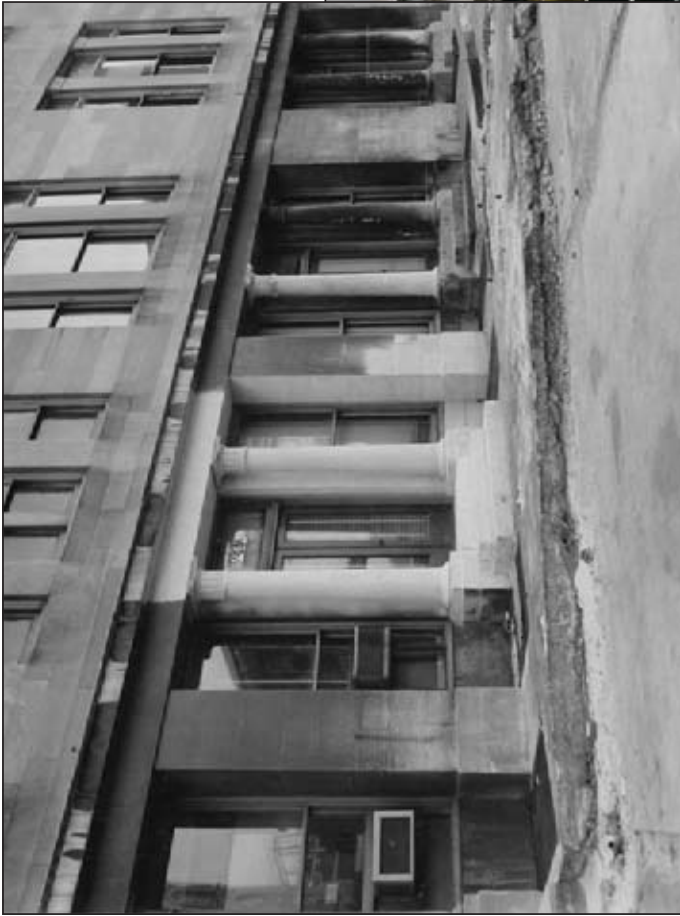
Figure 4.25: North Elevation, columns 5-10 Source: INHP Archives Date: December 2, 1953 Columns 5-6 was sandblasted, Column 7 was recarved
