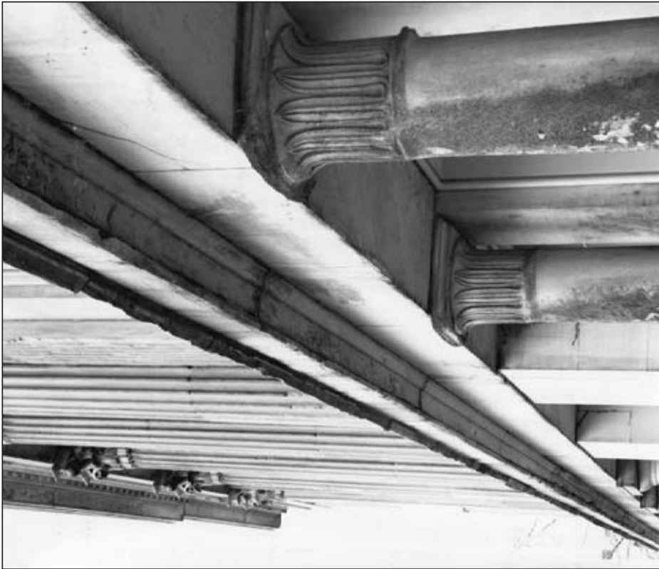
Figure 4.14: West Elevation, columns 3 and 4 Source: INHP Architects' office Creator: William Brookover Date: March 3, 1984
