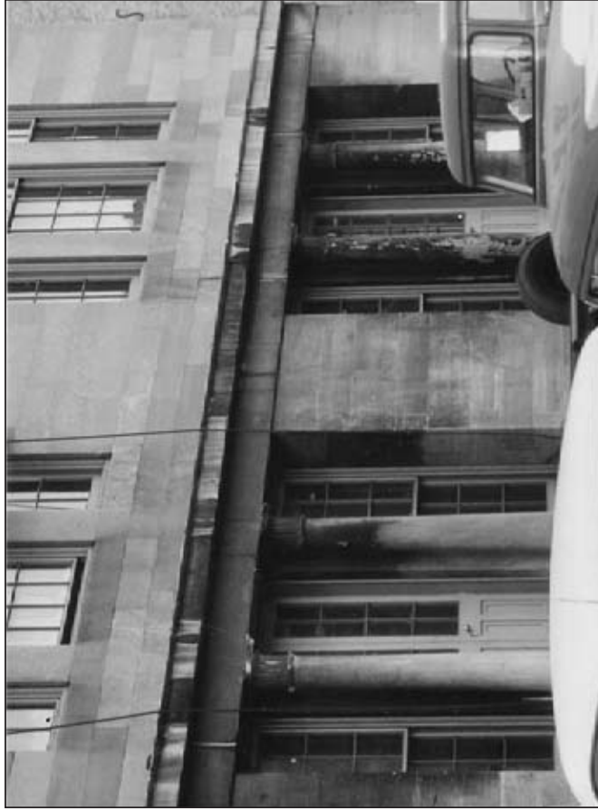
Figure 4.24: North Elevation, Columns 7-10 Source: INHP Archives Creator: W. A. McCullough Date: April 5, 1961
