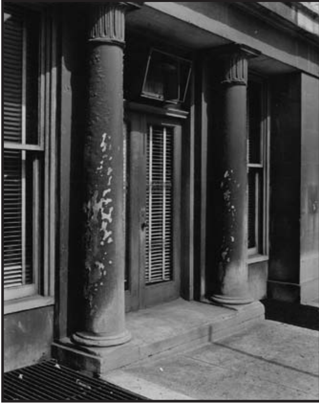
Figure C.50: South elevation, columns 3 and 4 Source: INHP Archives Caption: Merchants' Exchange: South wall, second entrance from west end. Detail showing disintegration of first floor marble columns Creator: Knickerbocker (Housam) Date: March 20, 1952
