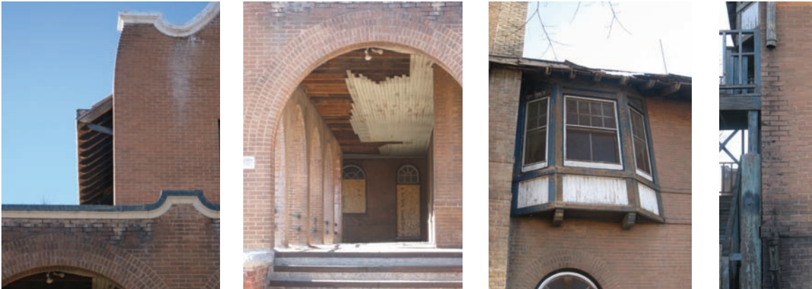
Figs 79-82 (l-r): La Castañeda currently suffers from mortar loss and roof drainage problems; threats to wood rafters; wood rot; and no gutter connections to move water away from the foundations.
