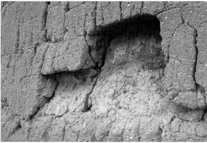
Figure 6. Lower west wall of the Casa Grande, north end showing area of detachment and loss in 1975 (left) and 1995 (right), 1998 (ACL).
