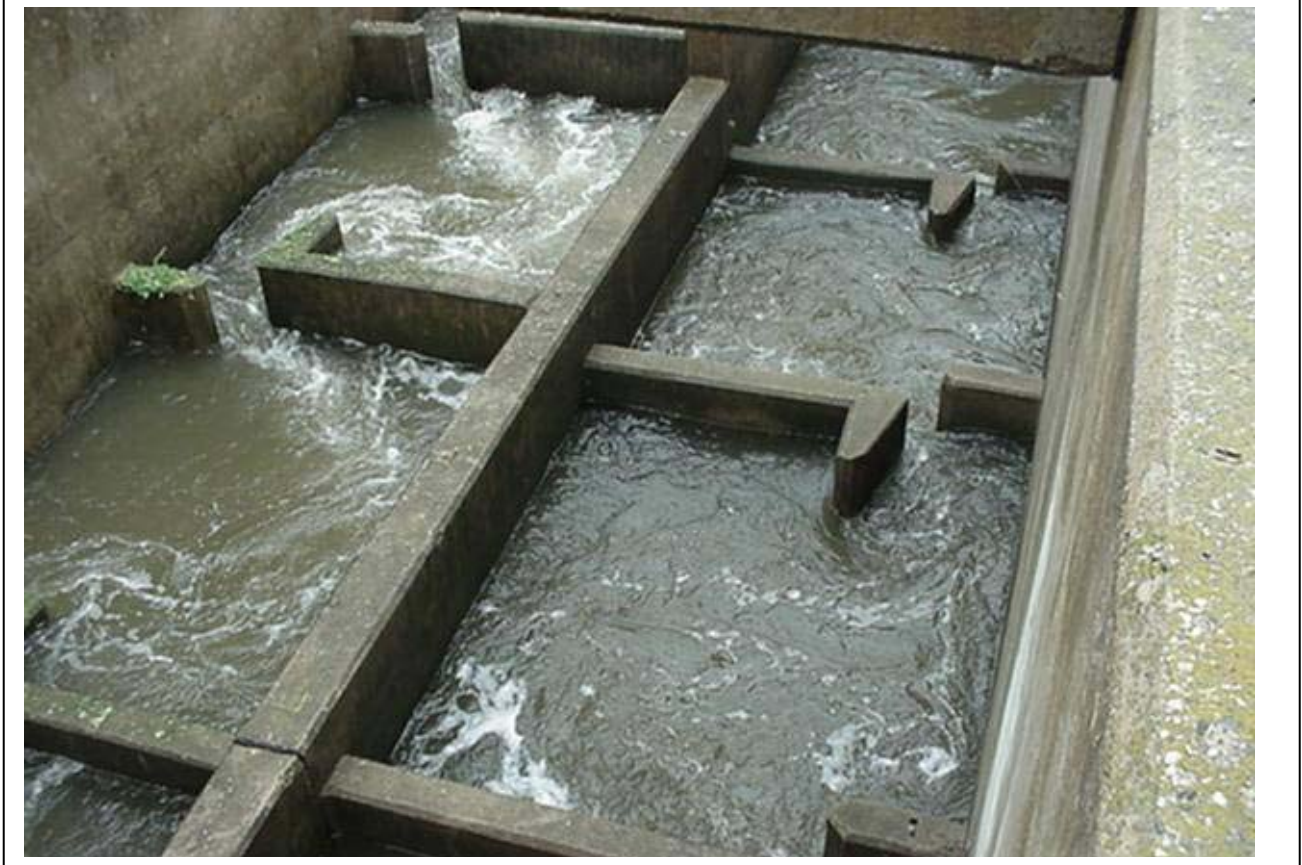
Figure 5. Overhead view looking into Fairmount fishway. Pools are formed by concrete walls and separated by baffles, which create vertical slots for fish to swim through. Fish will swim from one pool to another by passing through the slots, incrementally making their way to the top of the fishway and above the dam.
