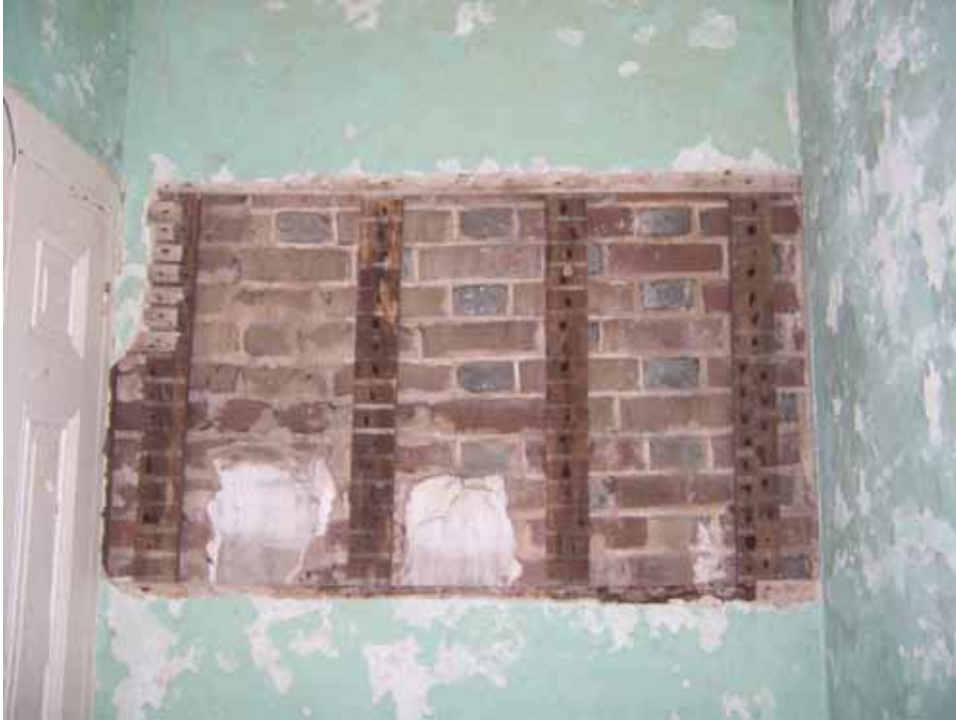
Figure 23. Photographic evidence of earlier attached kitchen addition on the west façade of the original building. (Source: A. Aiken; taken 10/12/2006.)
