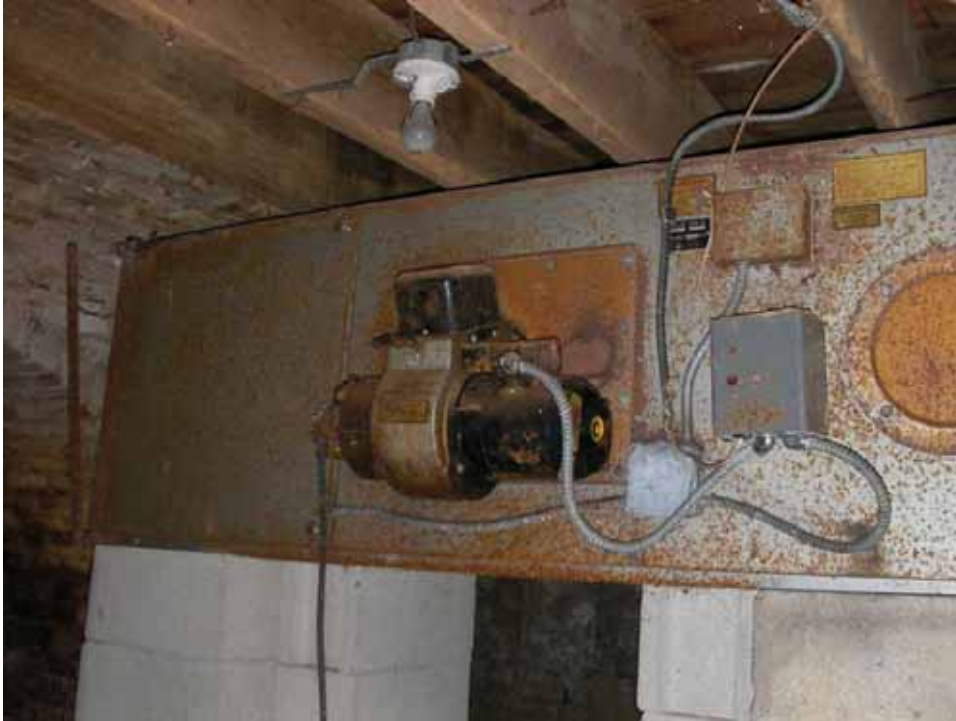
Figure 60. Photograph of the mechanical equipment in the west room of the 1859 addition block of the Abel and Mary Nicholson house. (Source: A. Aiken; taken 2/23/2007.)
