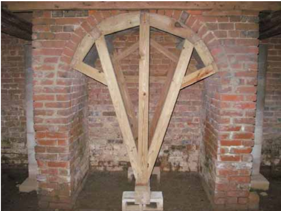
Figure 36. Photograph of the east room wooden reinforced arched brick chimney support on the east wall of the 1722 block of the Abel and Mary Nicholson house. (Source: A. Aiken; taken 2/23/2007.)
