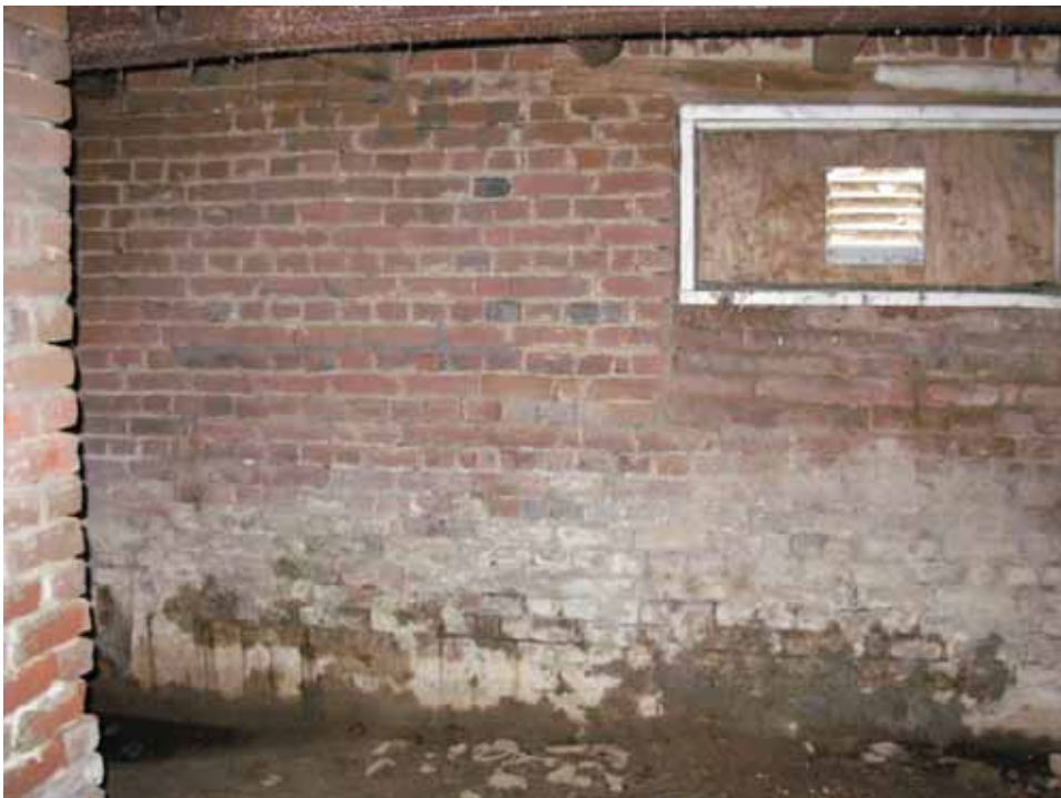
Figure 43. Photograph of the damp water staining at the bottom of the south wall of the east room in the 1722 block of the Abel and Mary Nicholson house. (Source: A. Aiken; taken 2/23/2007.)
