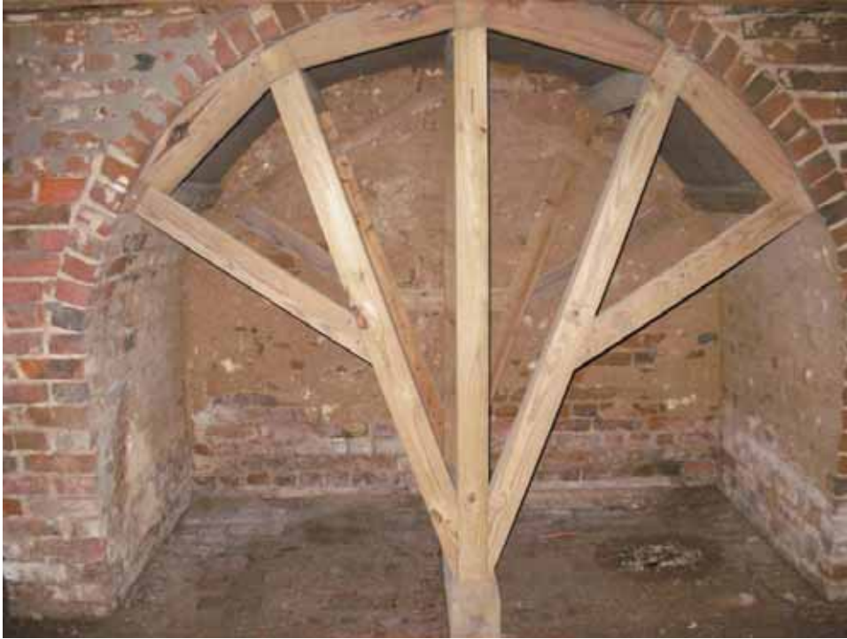
Figure 37. Photograph of the west room wooden reinforced arched brick chimney support on the west wall of the 1722 block of the Abel and Mary Nicholson house. (Source: A. Aiken; taken 2/23/2007.)
