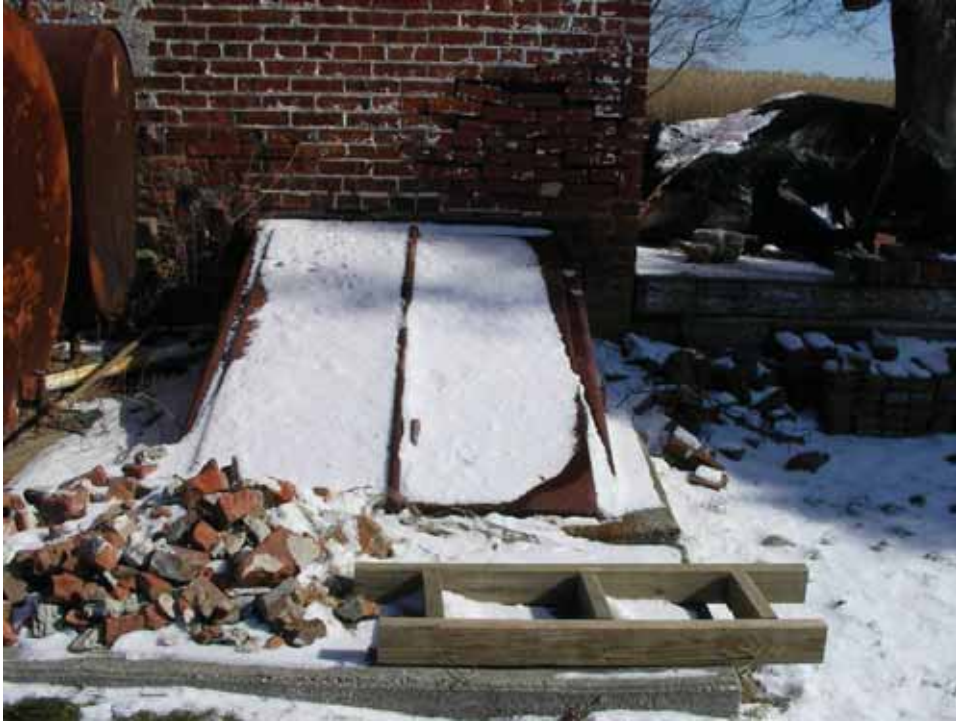
Figure 35. Photograph of the bulkhead door, on the west façade, that leads to the basement of the 1859 block of the Abel and Mary Nicholson house. (Source: A. Aiken; taken 2/7/2007.)
