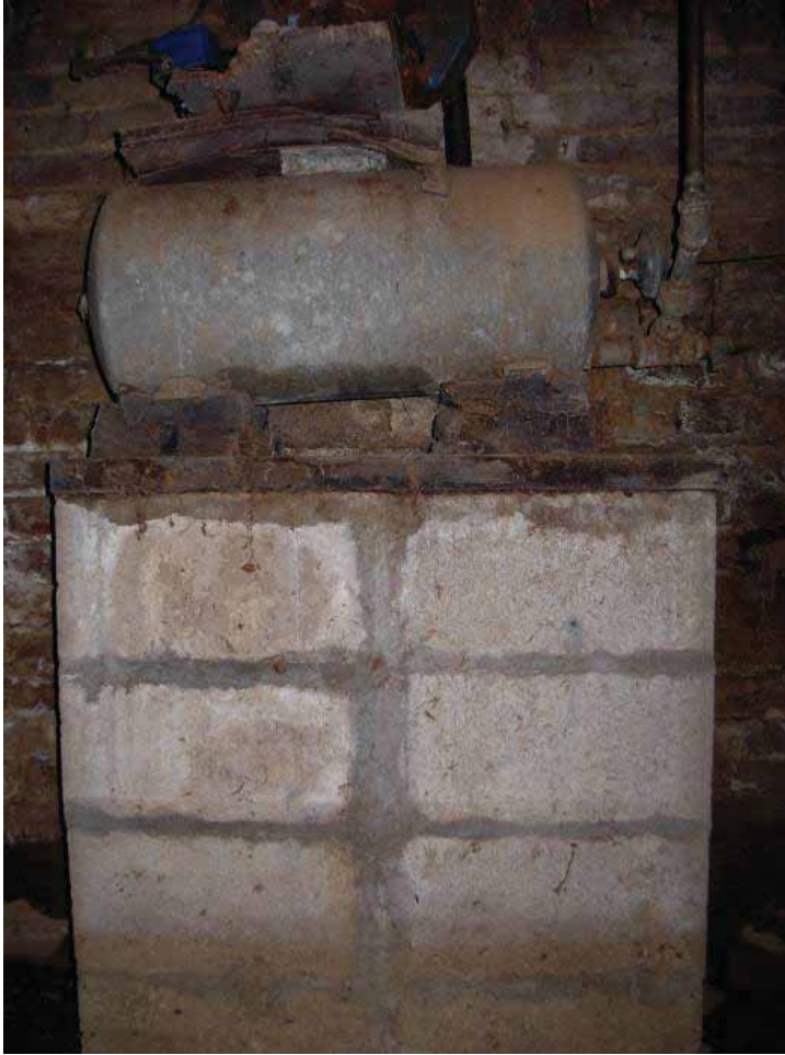
Figure 32. Photograph of the 12-gallon storage pressure water tank located on the south wall of the west cellar room in the 1859 block of the Nicholson house. (Source: A. Aiken; taken 2/23/2007.)
