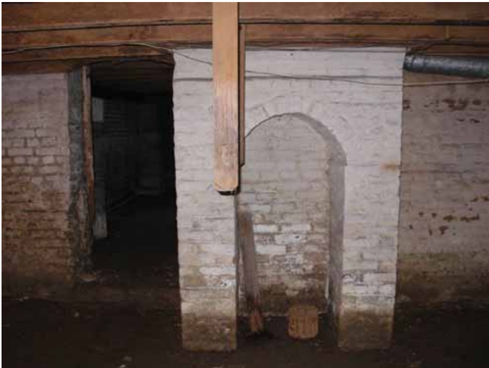
Figure 38. Photograph of the east room arched brick chimney support on the east wall of the 1859 block of the Abel and Mary Nicholson house. (Source: A. Aiken; taken 2/23/2007.)
