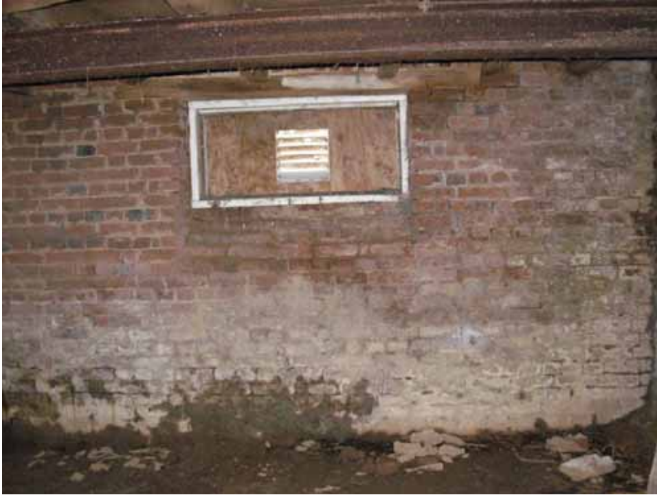
Figure 50. Photograph of the south cellar wall in the east room of the 1722 block of the Abel and Mary Nicholson house. (Source: A. Aiken; taken 2/23/2007.)
