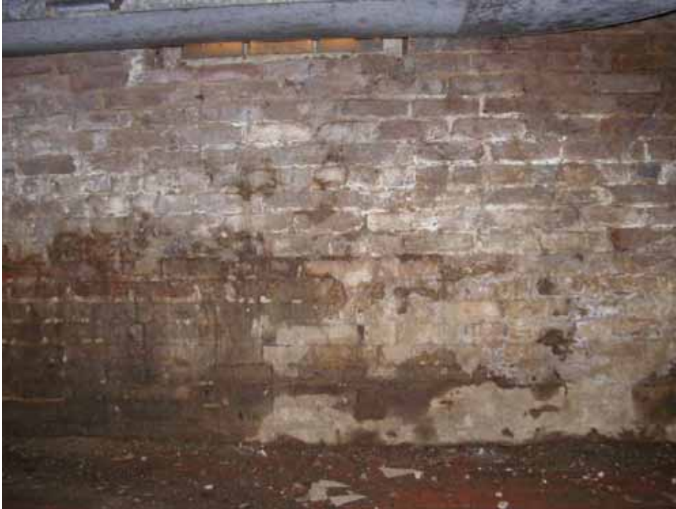
Figure 46. Photograph of the discoloration of the south brick cellar wall next to the water staining, near the ground of the 1859 block west room of the Abel and Mary Nicholson house. (Source: A. Aiken; taken 2/23/2007.)
