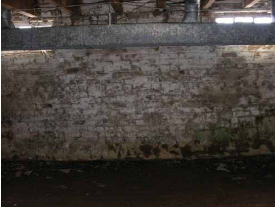
Figure 58. Photograph of the south wall and ductwork in the east room of the 1859 addition block of the Abel and Mary Nicholson house. (Source: A. Aiken; taken 2/7/2007.)
