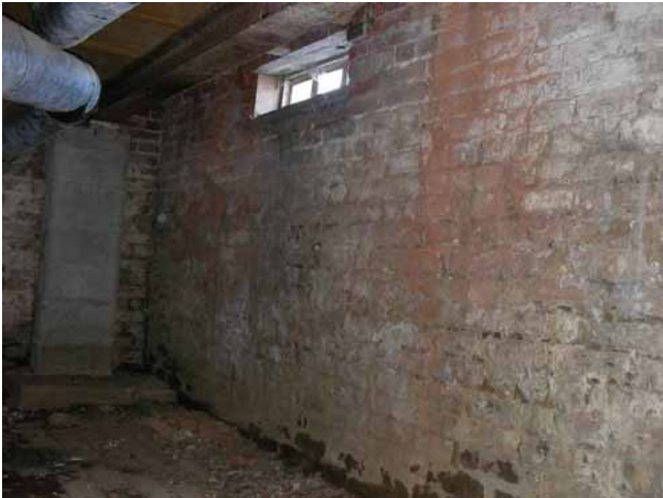
Figure 57. Photograph of the north wall of the west room of the 1859 addition block of the Abel and Mary Nicholson house. (Source: A. Aiken; taken 2/7/2007.)
