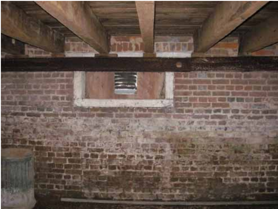
Figure 49. Photograph of the north cellar wall in the west room of the 1722 block of the Abel and Mary Nicholson house. (Source: A. Aiken; taken 2/23/2007.)
