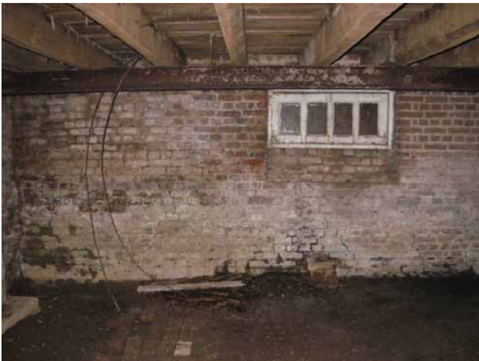
Figure 47. Photograph of the white discoloration of the south brick cellar wall near the ground and under the window of the 1722 block west room of the Abel and Mary Nicholson house. (Source: A. Aiken; taken 2/23/2007.)
