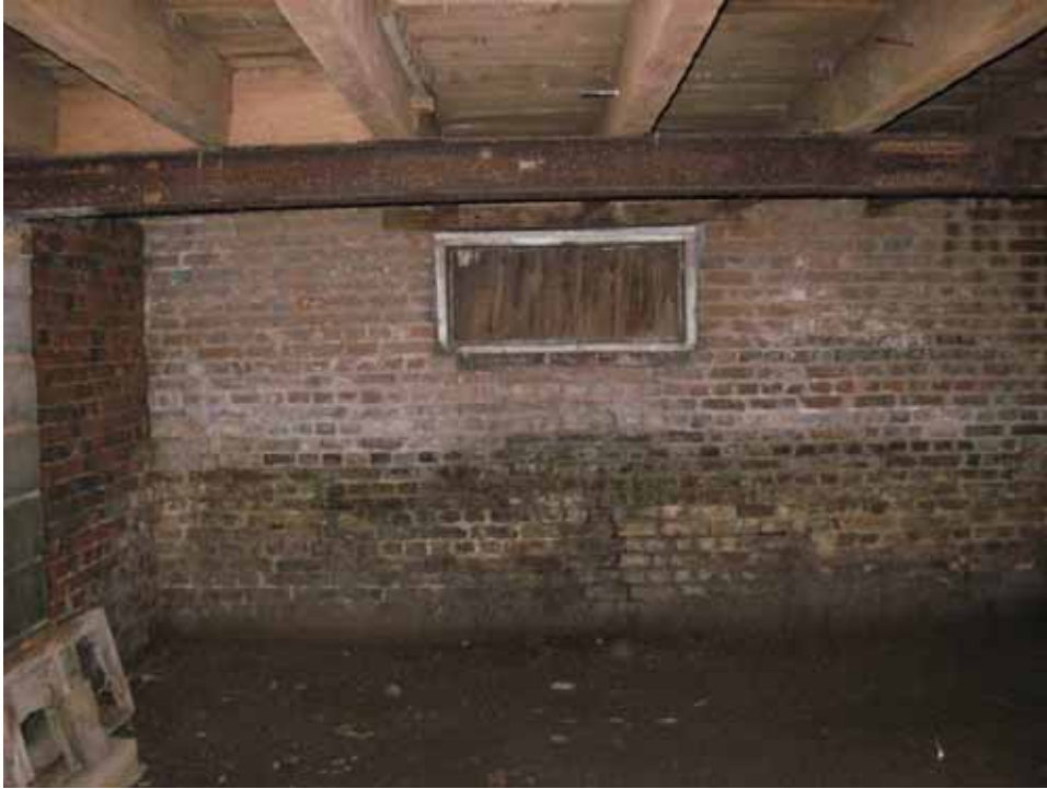
Figure 48. Photograph of the north cellar wall in the east room of the 1722 block of the Abel and Mary Nicholson house. (Source: A. Aiken; taken 2/23/2007.)
