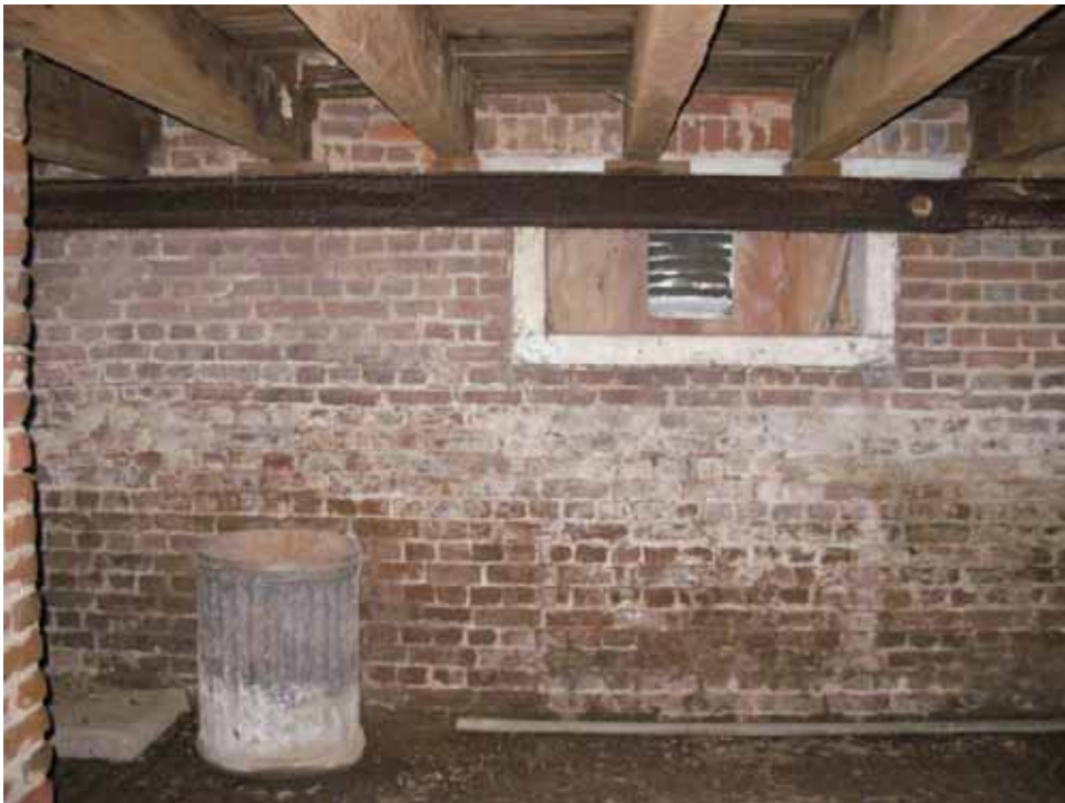
Figure 45. Photograph of the dark discoloration of the north brick cellar wall near the ground of the 1722 block west room of the Abel and Mary Nicholson house. (Source: A. Aiken; taken 2/23/2007.)
