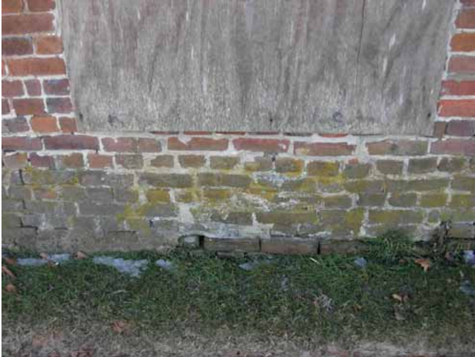
Figure 44. Photograph of the green staining and poor brick and mortar conditions at the bottom, east corner of the north facade of the 1722 block of the Abel and Mary Nicholson house. (Source: A. Aiken; taken 2/23/2007.)
