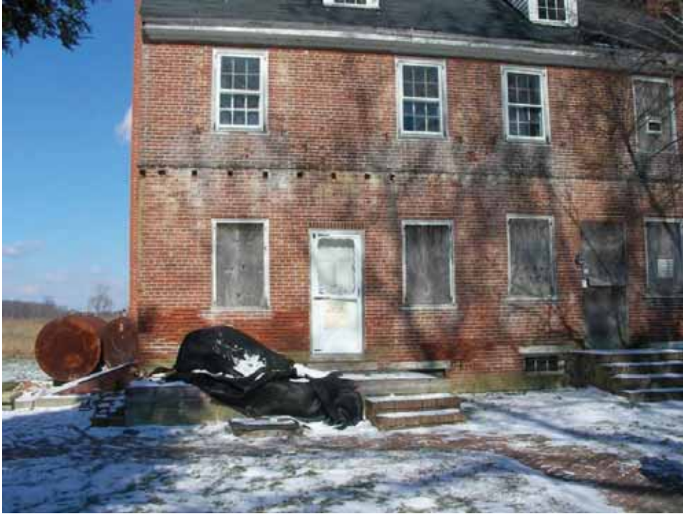
Figure 26. Photograph of today's main entrance on the south façade of the 1859 block of the Abel and Mary Nicholson house. (Source: A. Aiken; taken 2/7/2007.)
