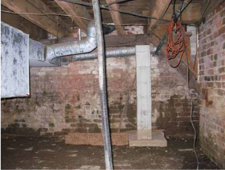
Figure 56. Photograph of the north wall of the west room of the 1859 addition block of the Abel and Mary Nicholson house. (Source: A. Aiken; taken 2/23/2007.)
