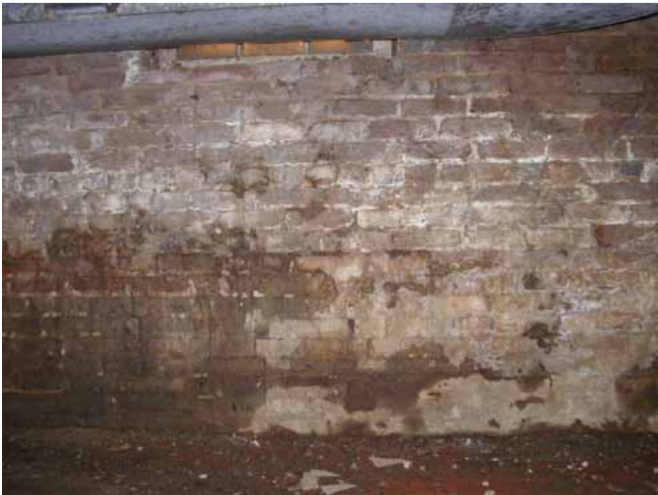
Figure 59. Photograph of the south wall and west room of the 1859 addition block of the Abel and Mary Nicholson house. (Source: A. Aiken; taken 2/23/2007.)
