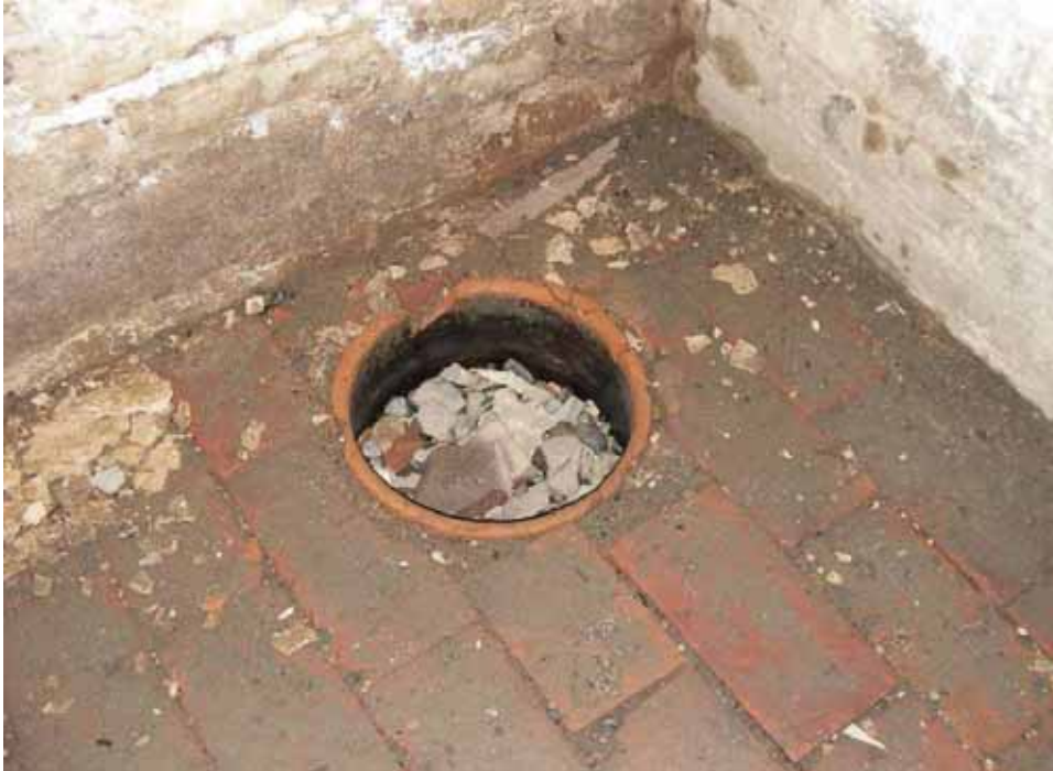
Figure 62. Photograph of a red cylindrical pipe possibly intended for drainage in the east room of the 1859 addition block of the Abel and Mary Nicholson house. (Source: A. Aiken; taken 2/7/2007.)
