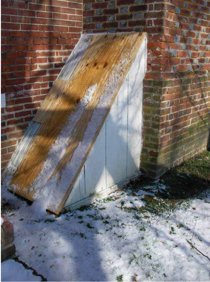
Figure 34. Photograph of the bulkhead door, on the south façade, that leads to the basement of the 1722 block of the Abel and Mary Nicholson house. (Source: A. Aiken; taken 2/7/2007.)
