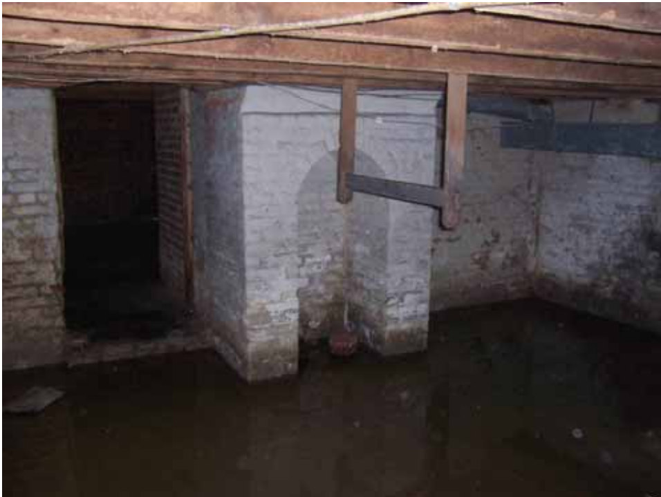
Figure 41. Photograph of the flooded cellar from the cellar staircase, looking into the 1859 block east room of the Abel and Mary Nicholson house. (Source: A. Aiken; taken 10/12/2006.)
