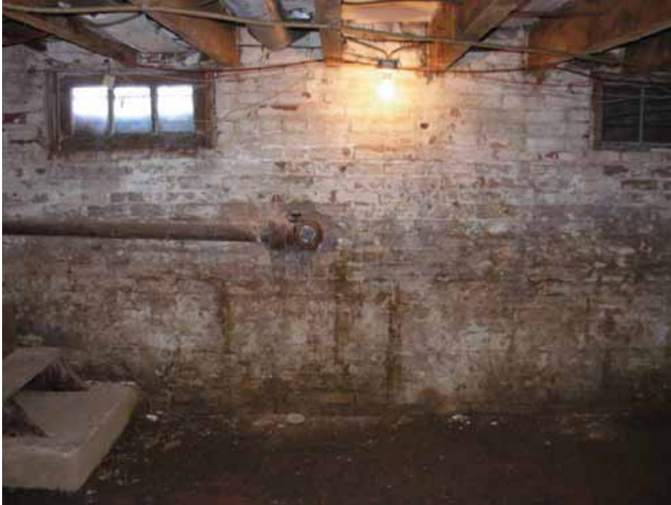
Figure 40. Photograph of the fading whitewash coating on the north wall of the 1859 block east room of the Abel and Mary Nicholson house. (Source: A. Aiken; taken 2/23/2007.)
