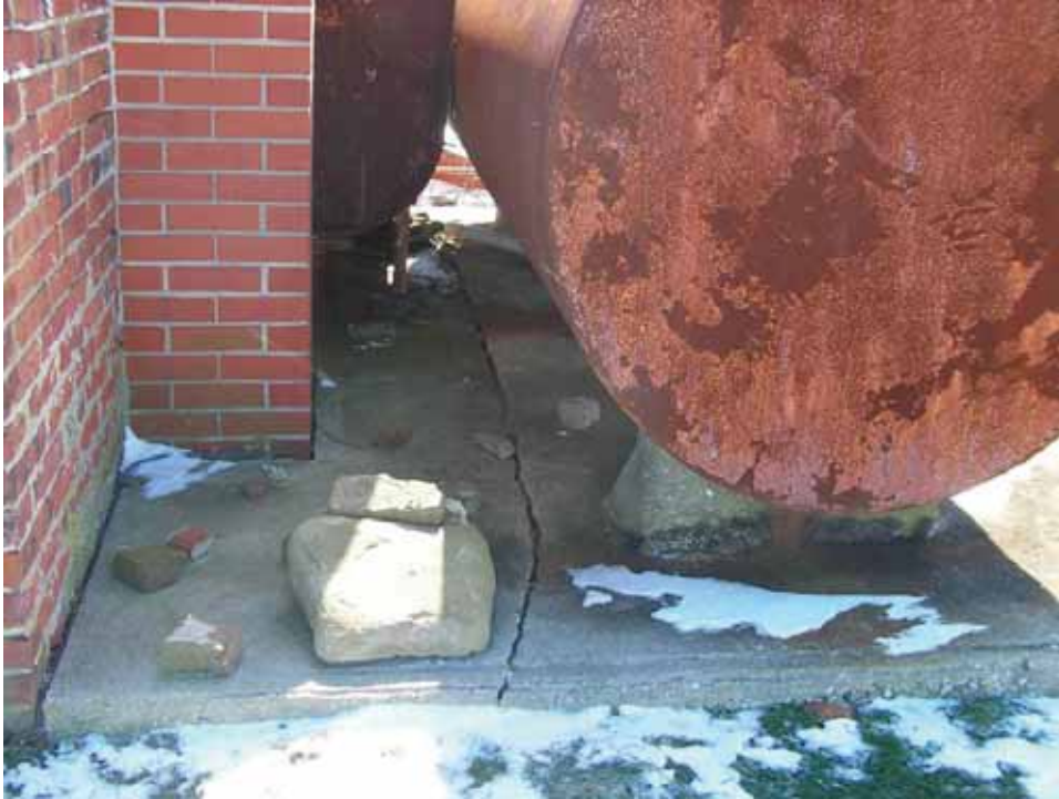
Figure 30. Photograph of the major crack in the concrete pad supporting the oil storage tank on the west façade of the Nicholson house. (Source: A. Aiken; taken 2/7/2007.)
