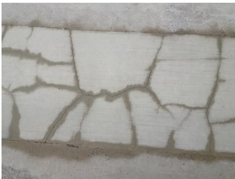
Figure 78: Cracked patch that was placed with no curing
