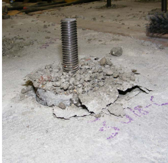
Figure 4-3 Failed core pullout specimen
