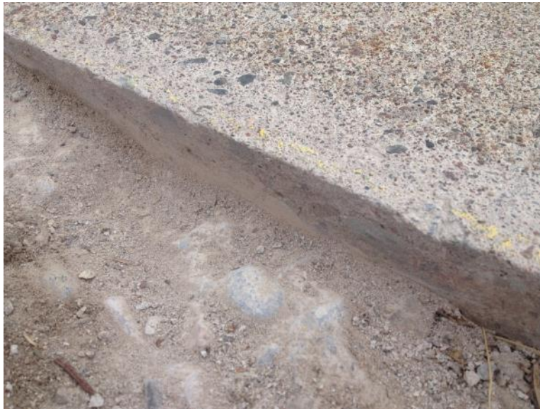
Figure 74: Saw-cut edge of a patch area, vertical face
