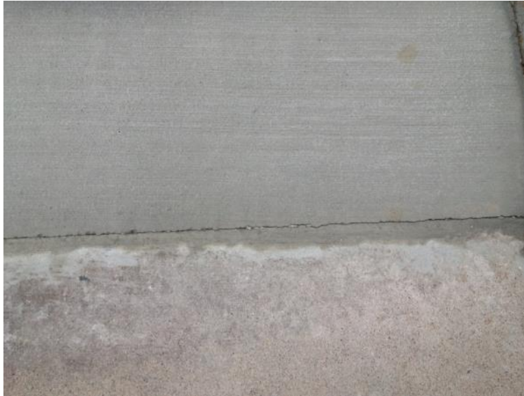
Figure 76: Edge de-bonding due to shrinkage along a saw-cut patch area
