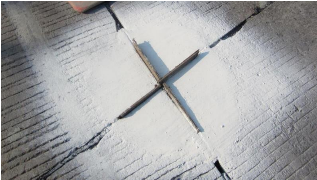
Figure 88: A finished patch with fiber board inserted to maintain a working joint
