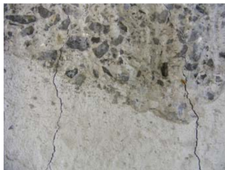
(c) Cracking underneath patch area
