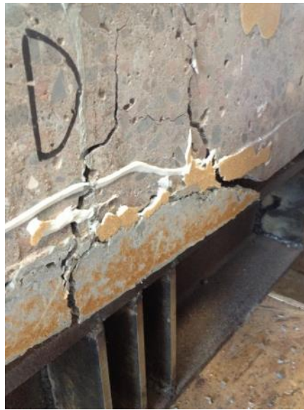
Figure 65: Specimen “D” (D3-2-G) started cracking at the edge of the patch, the bond held and the slab failed in two locations.
