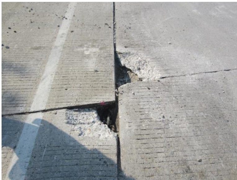
Figure 75: Tapered edges of two opposing corner partial-depth repairs
