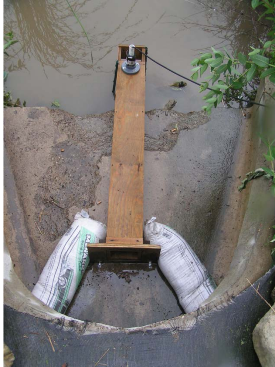
Figure 5.6. Turbidity box mounted in culvert outfall from sediment pond
