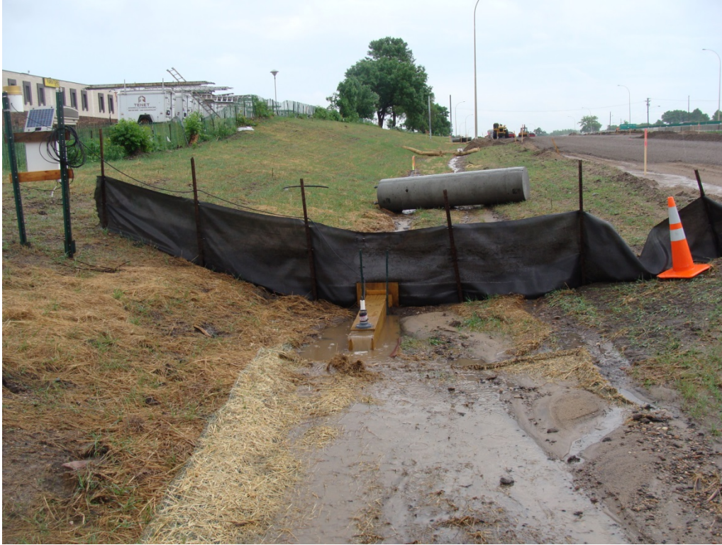
Figure 5.23. Turbidity monitoring setup at 169/494 after rainfall event
