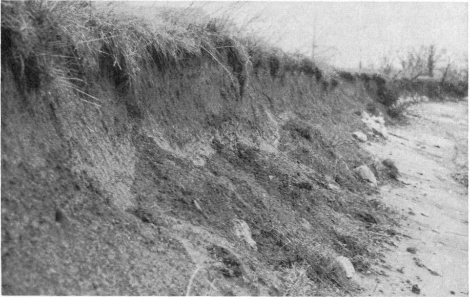
FIGURE 12. Crumb-mulch talus slumped by rainfall. February 16, 1949.
