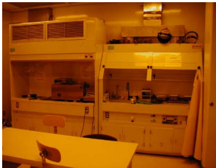
Figure 3.3: Wet bench for wafer cleaning
