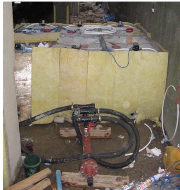
Figure 2. Plastic insulated containers for heated water storage
