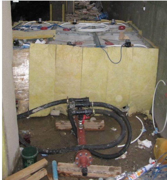
Figure 9-9 Plastic insulated containers for heated water storage
