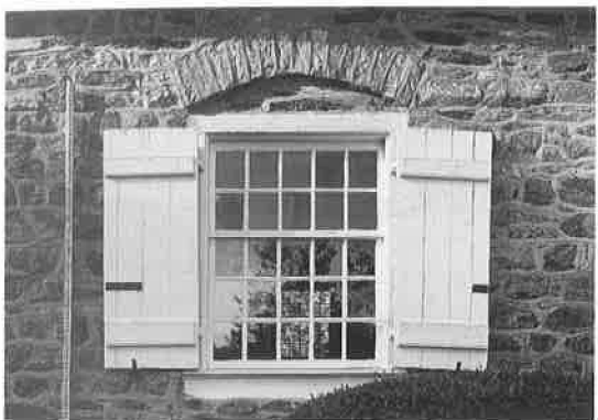
Detail of window at the south front facade of Radnor Meetinghouse. (Jack E. Boucher, photographer, 1998.)
