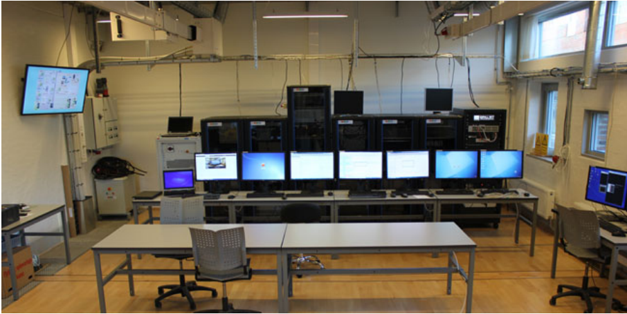
Fig. 2.6: Picture of the Smart Energy Systems Laboratory at Aalborg University [12].
