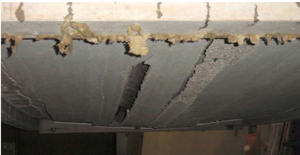
Figure 8. Damages after 25 minutes. Photo K. Hertz.
