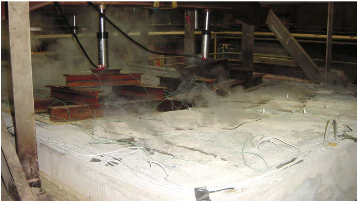
Figure 7. Cracks in top flange after approx. 15 min. Photo K. Hertz.
