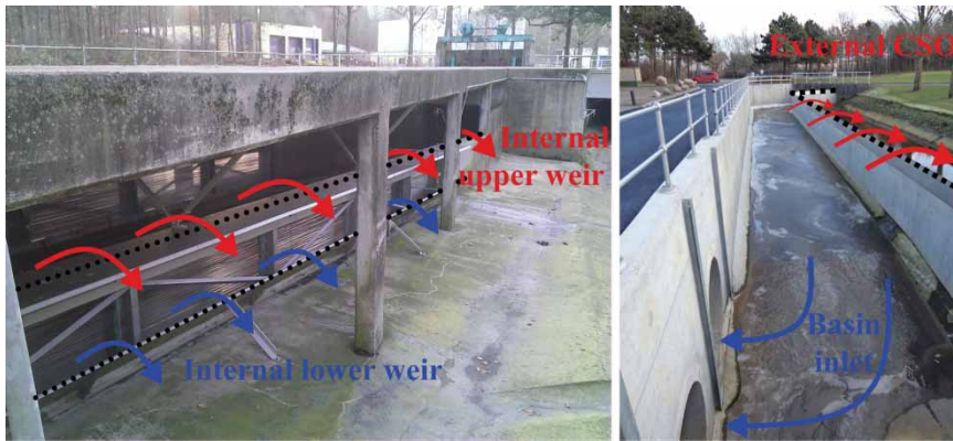
Figure 4 | Photograph of the internal and external CSO during dry weather. The left photograph is taken from the north-eastern side of the internal CSO structure. The internal CSO is symmetric along the centreline of the inflow channel. The right photograph is taken from the western side of the external CSO structure.
