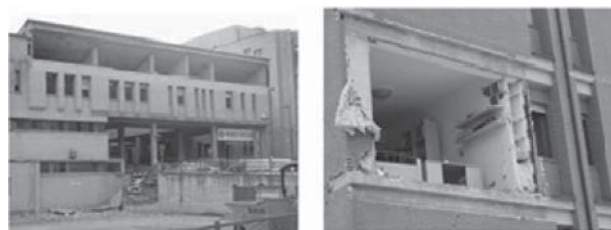
Figure 1. Damage in non-structural elements (Braga et al., 2011).
