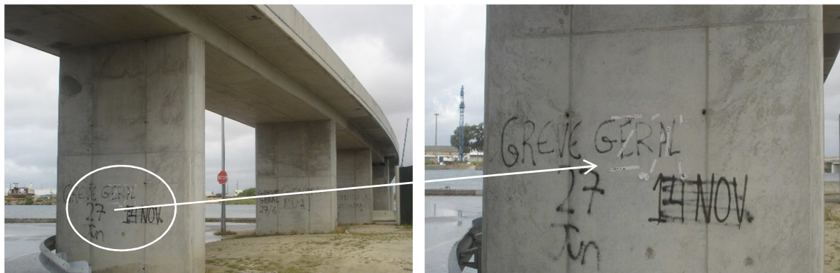
Fig. 1. Fair-faced concrete with graffiti , Bridge of Canal do Boco, Ílhavo (2014).
