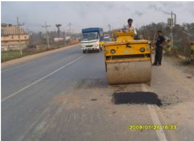
Plate 7.12: Reinstatement of bituminous layer is in progress by bituminous materials in pit at N4 road.
