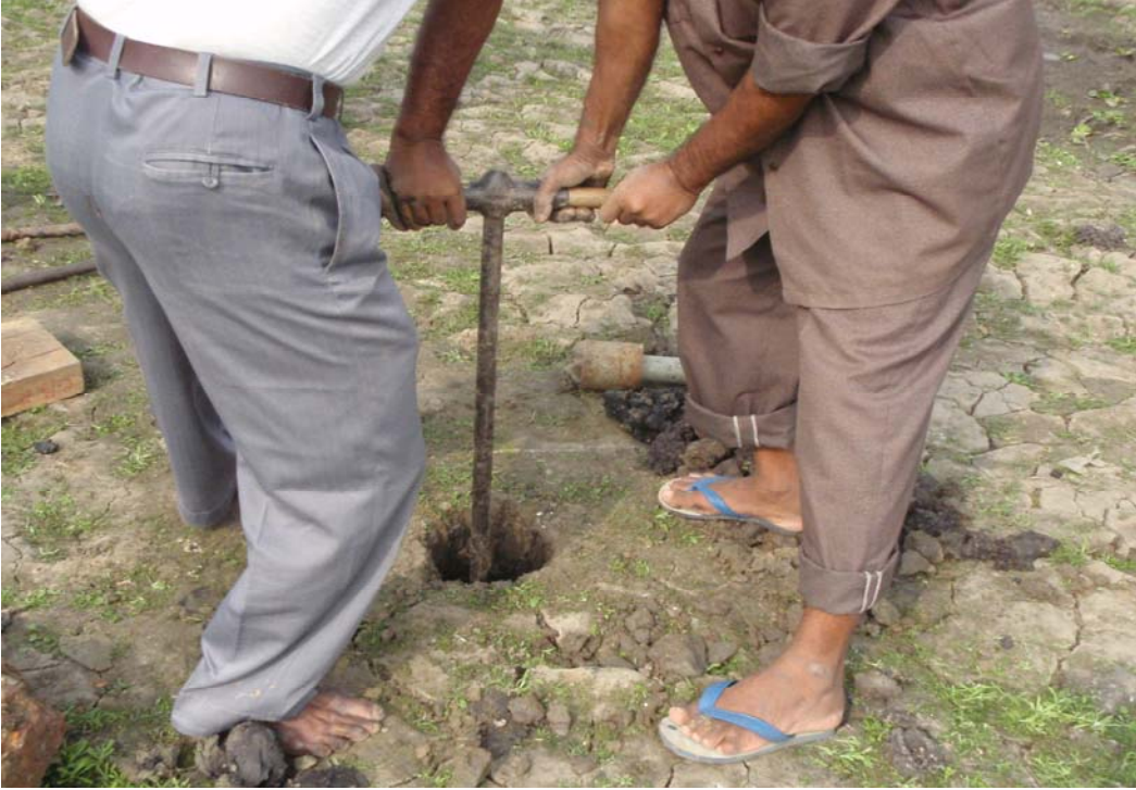
Plate 7.1: Boring is in Progress by Hand Auger at Tongi – Ashulia – EPZ Road embankment.
