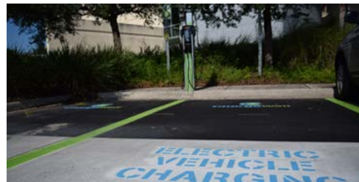
UNF'S FIRST ELECTRIC VEHICLE CHARGING STATION INSTALLED AT UNF HICKS HALL
