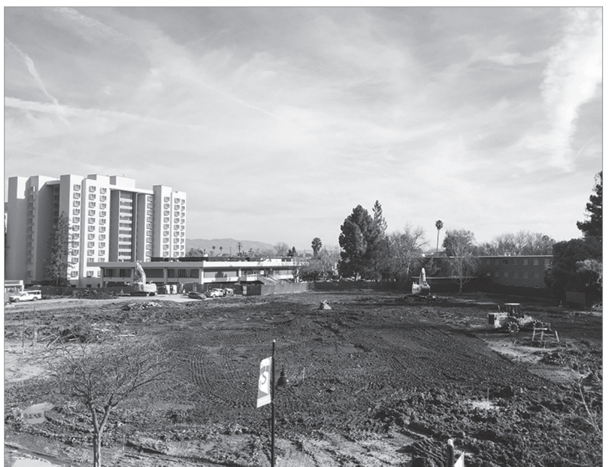
The aftermath of "The Bricks" dormitories being demolished to make room for the new aquatic center.
