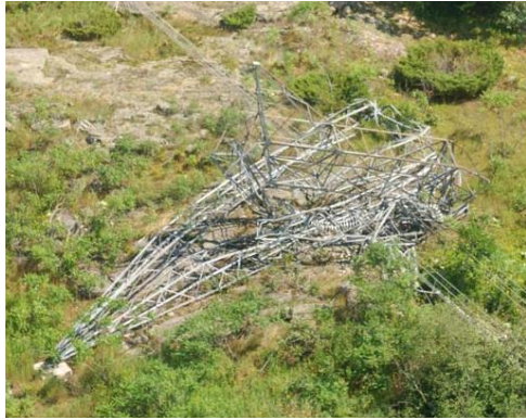
Fig. 3-1. Guyed tower failure (Hydro One report, 2006)
