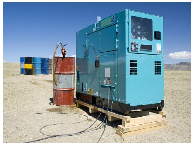
Figure 2 The standard diesel power generating system for a base station site [Hjorth et al. 2008].
