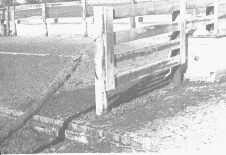
Spillage from waterers led to some erosion of fill adjacent to the concrete aprons.
