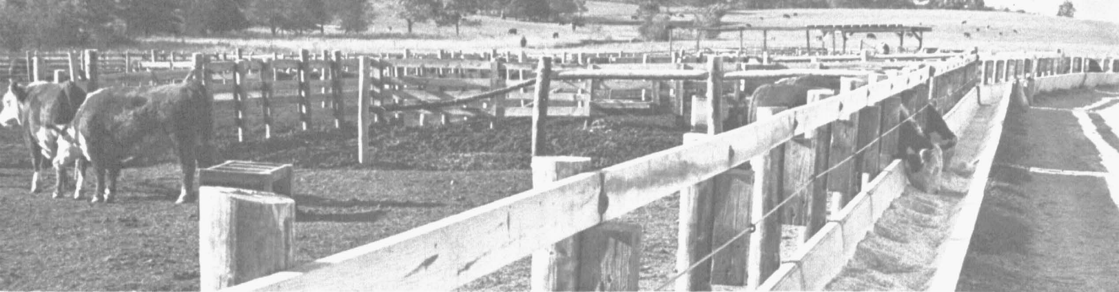
Precast concrete feed bunks were set in position with a wench truck.
