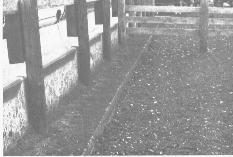
Erosion of fill resulting from too narrow apron presents an awkward situation (lot 6).
